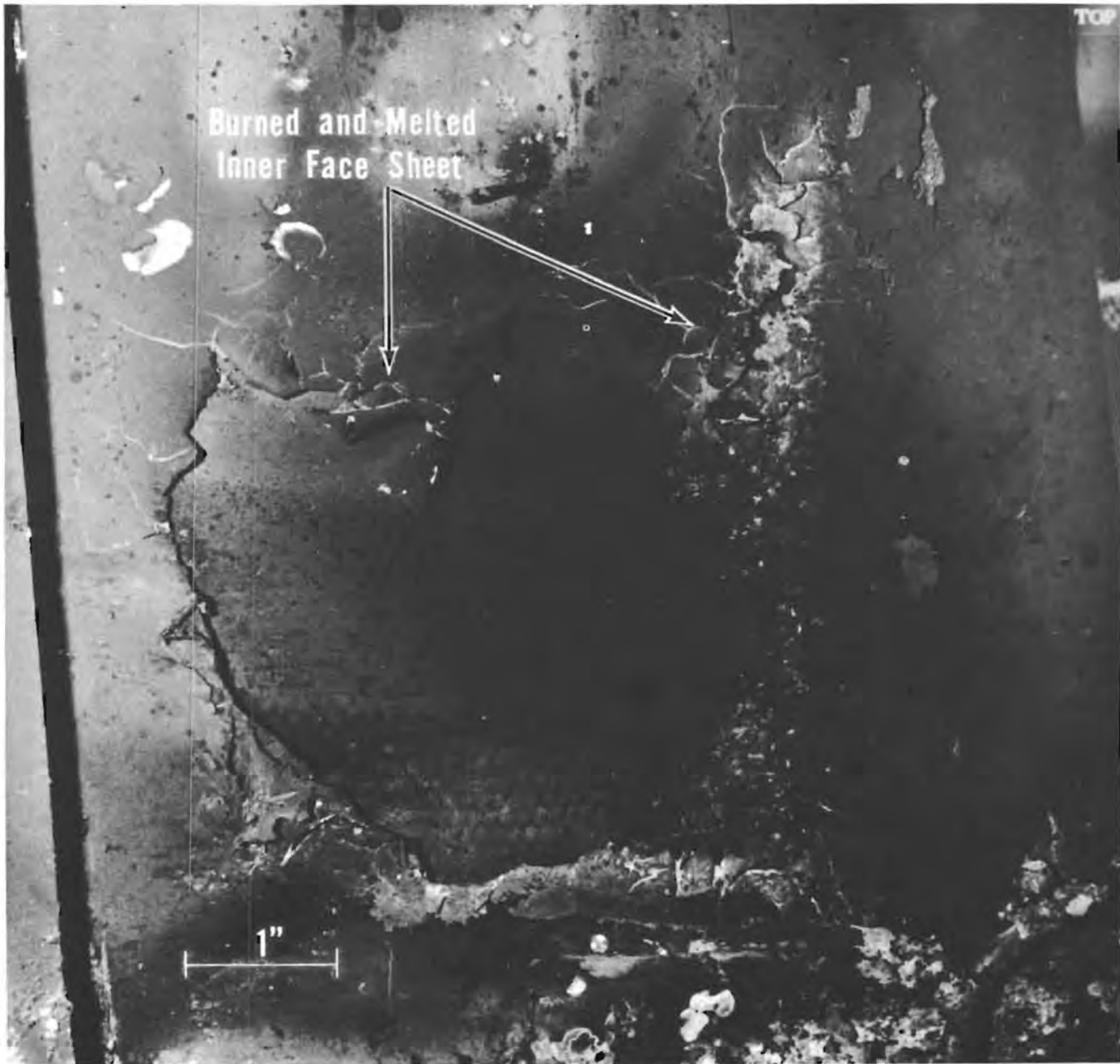
DAMAGED INNER SIDEWALL BELOW CO 2 ABSORBERS
