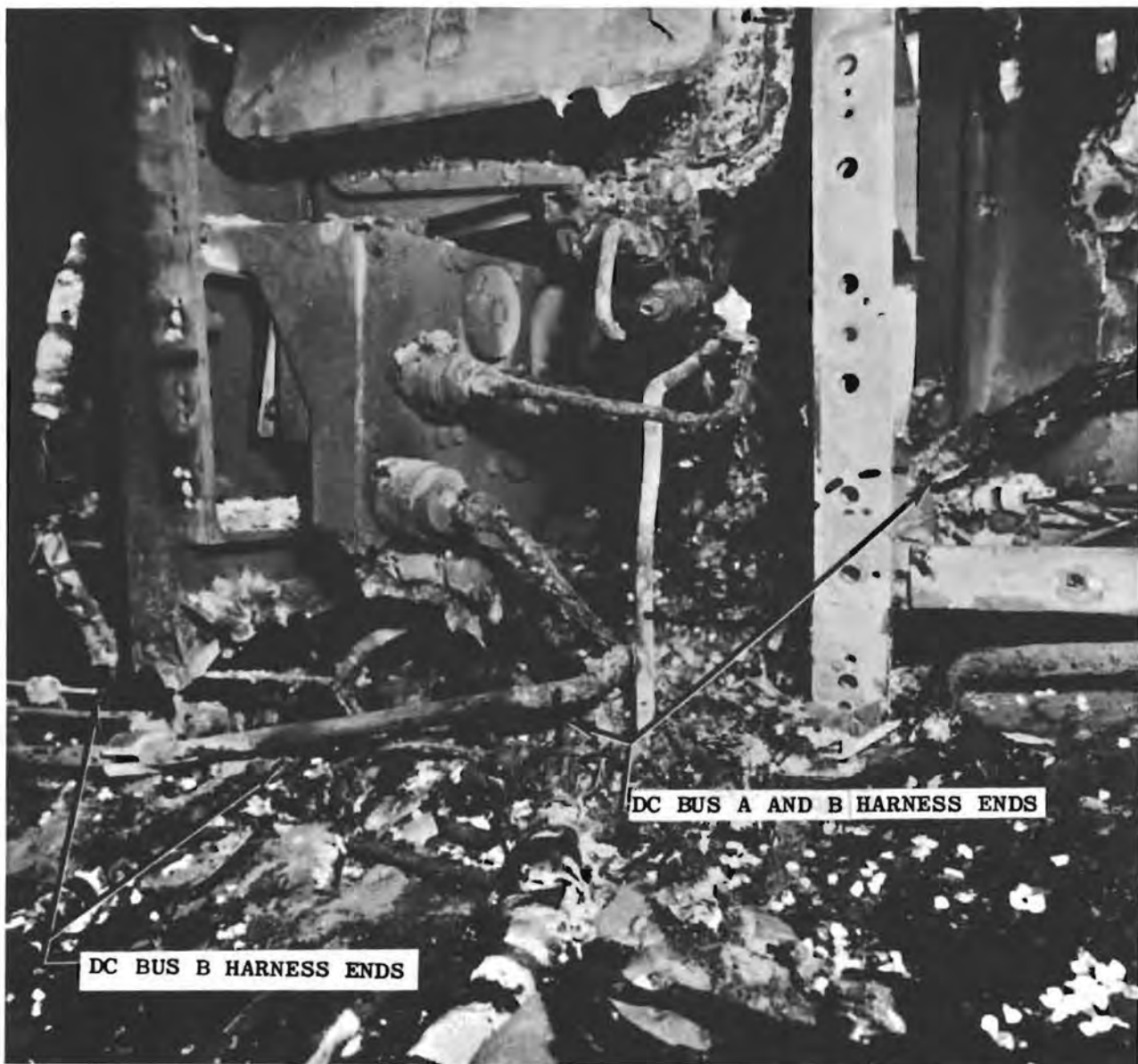
ENVIRONMENTAL CONTROL SYSTEM INSTRUMENTATION HARNESSES AFTER ACCIDENT
