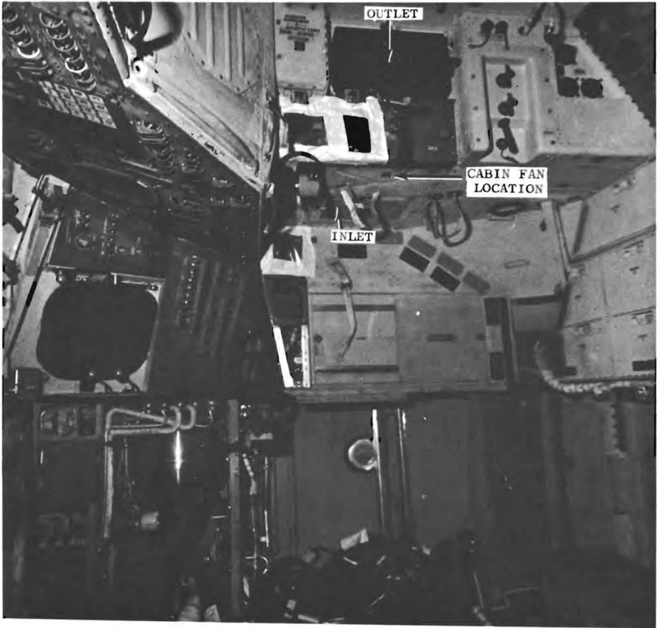
LOCATION OF CABIN FANS
