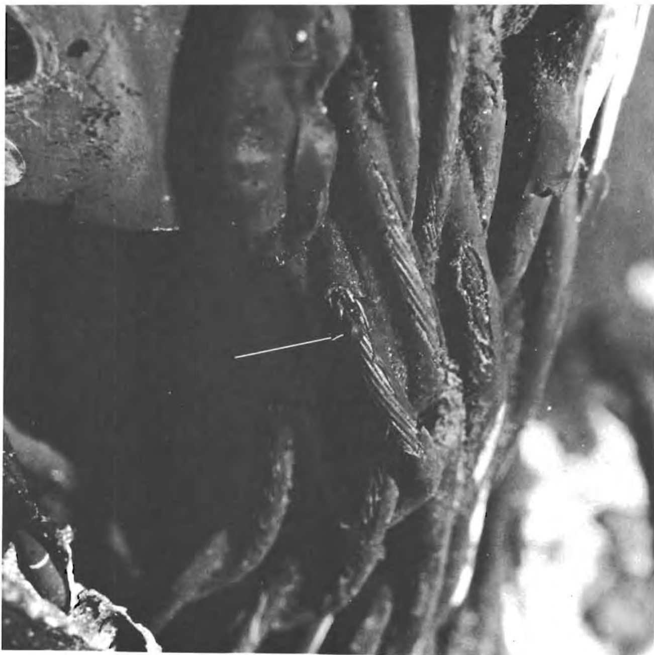
ARC POINT ON WIRE RELATED TO COVER OF JUNCTION BOX C15-1A52
