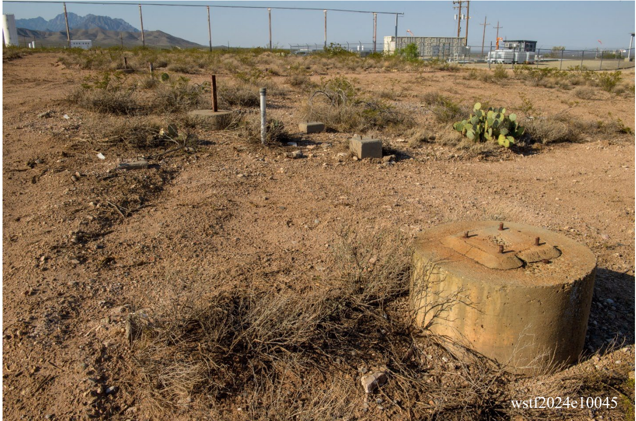
Figure 5 – Concrete pads with anchor bolts are the base mount of the burner and stack, and the white pipe is the electrical conduit. The metal stands on concrete were the piping mounts.
