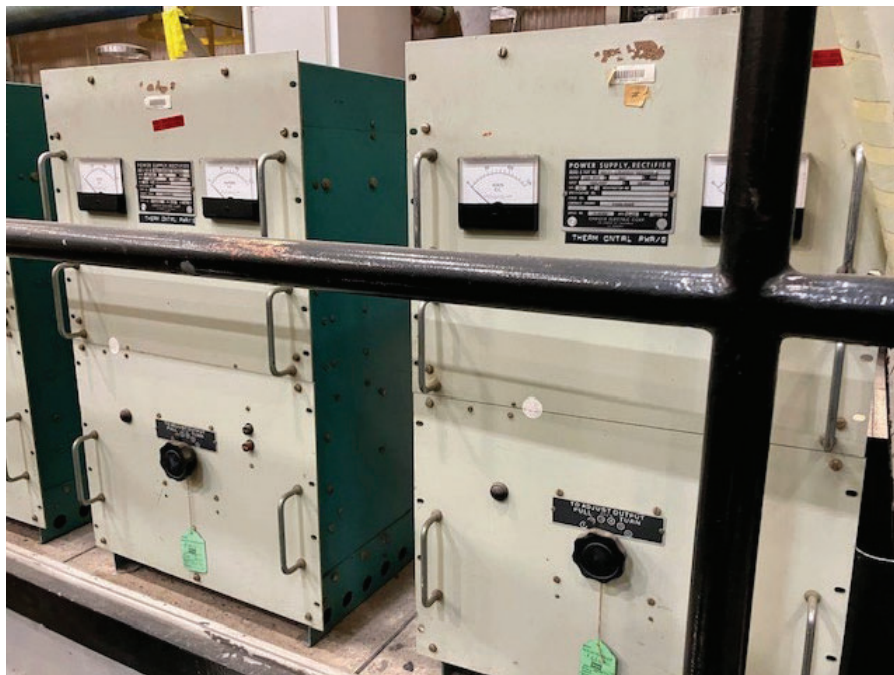
Figure 12. Front view of thermal control power transformers at Chamber B to be removed and excessed.
