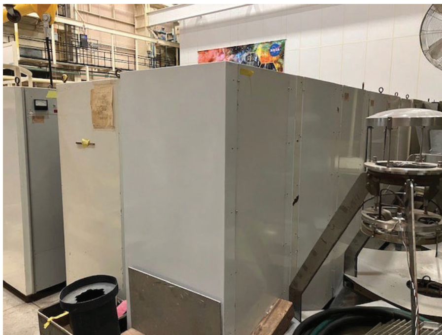
Figure 24. Additional miscellaneous obsolete equipment stored on platform to be removed and excessed.
