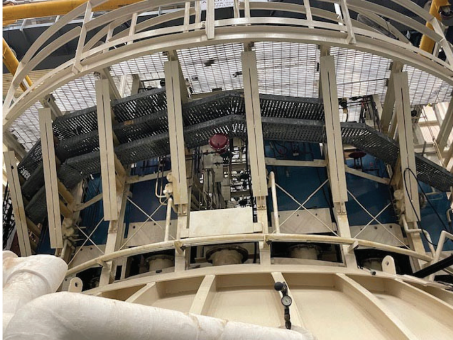
Figure 9. Metal cable trays (dark colored) below Chamber B catwalk to be removed and excessed.
