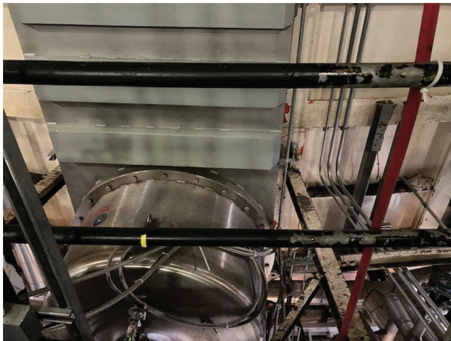
Figure 4. Top view for reference of cryopump installed on Chamber A.
