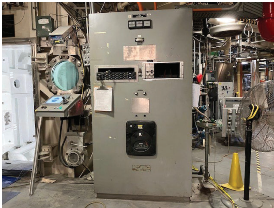
Figure 20. Additional peripheral control consoles for Chamber B to be removed and excessed.
