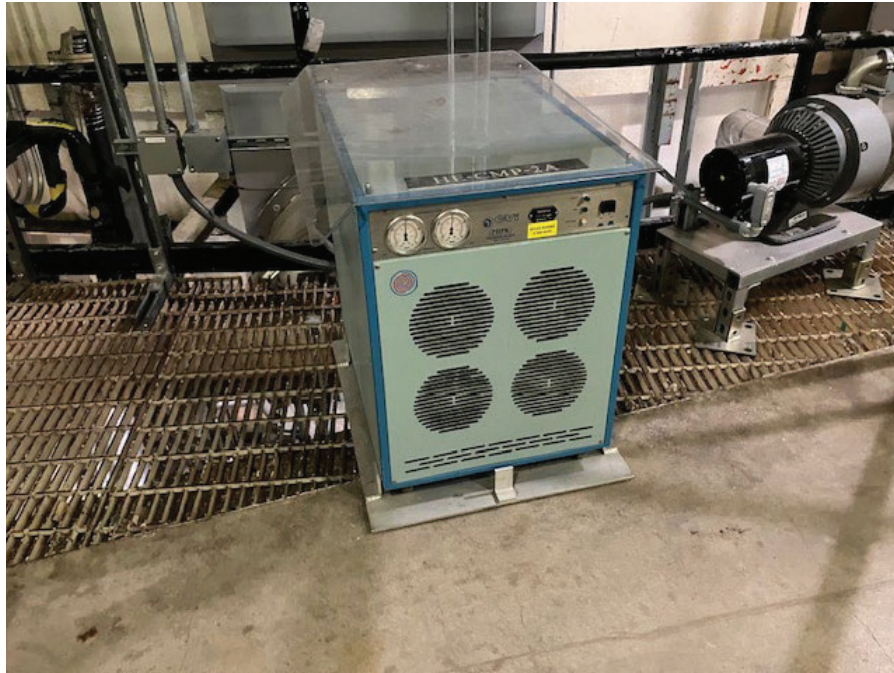
Figure 3. Example for reference of turbo pump controls at Chamber A.
