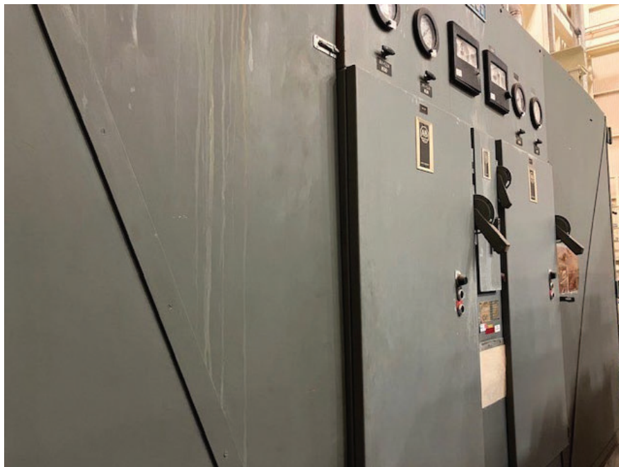
Figure 14. Supporting chiller for Chamber B to be removed and excessed.
