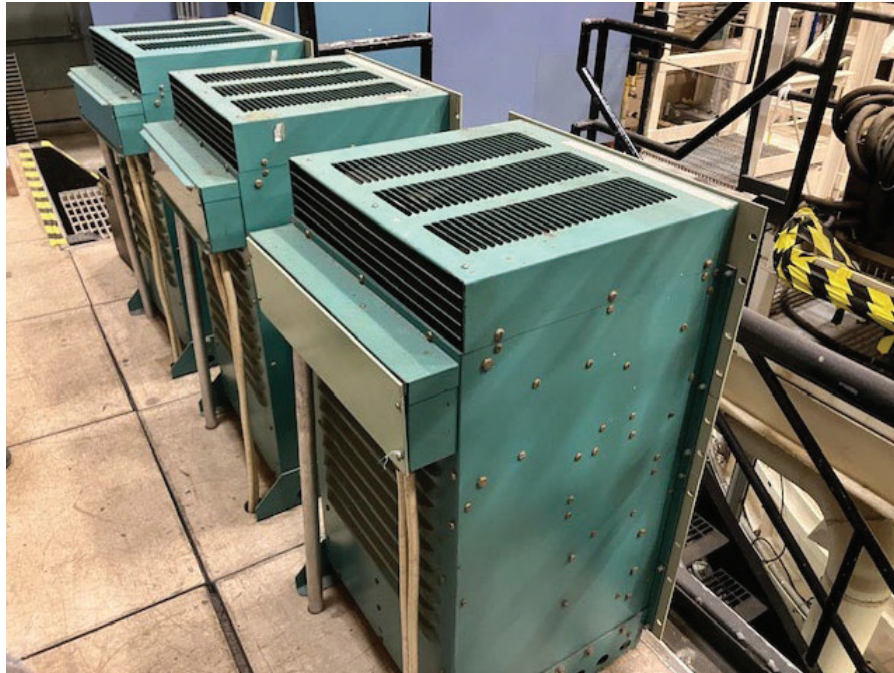
Figure 13. Back view of thermal control power transformers at Chamber B to be removed and excessed.
