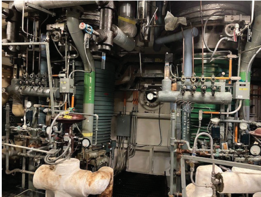
Figure 1. Two of the twelve diffusion pumps surrounding Chamber B to be removed and excessed, with chamber wall and viewing window visible behind.
