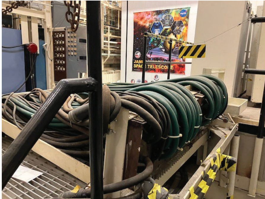
Figure 11. Cabling associated with solar simulators on Chamber B to be removed and excessed.
