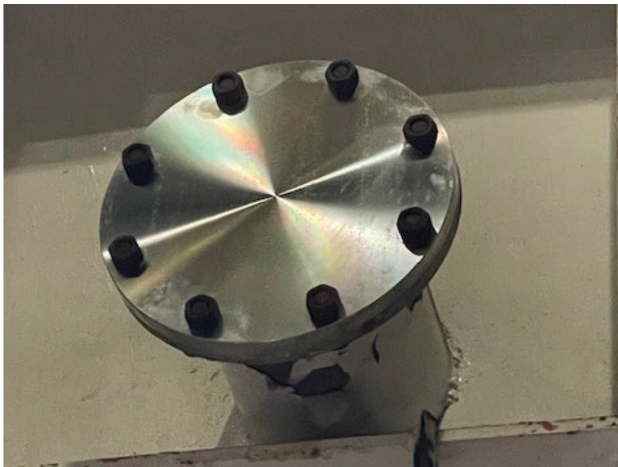
Figure 28. Metal cover installed to cover existing penetration on Chamber A, for reference.
