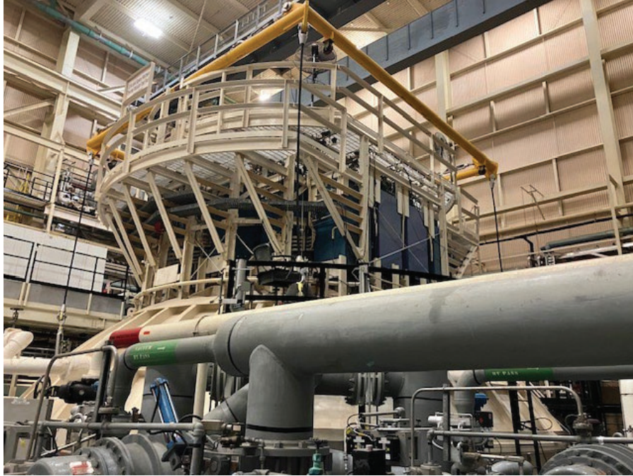
Figure 25. White metal catwalk on top of Chamber B to remain in place (blue solar simulators visible).
