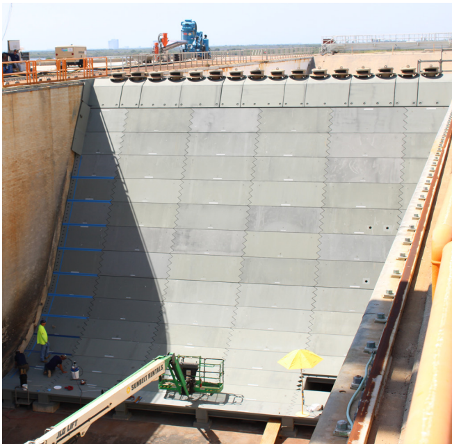
Steel plates make up the flame deflector inside the flame trench of pad 39B. (NASA) ▲
