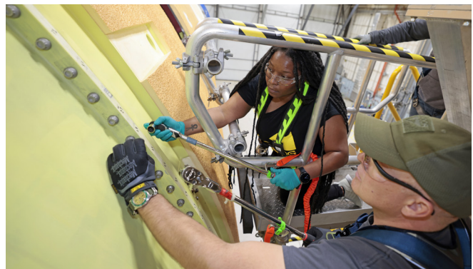
Engineers at Michoud insert 360 bolts to connect the forward assembly to the liquid hydrogen tank, making up the bulk of the core stage. (NASA) ▲
