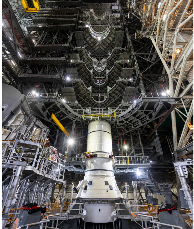
Engineers and technicians with EGS stack the left-aft assembly for the Artemis II SLS solid rocket booster onto mobile launcher 1 inside the VAB. (NASA) ▲
