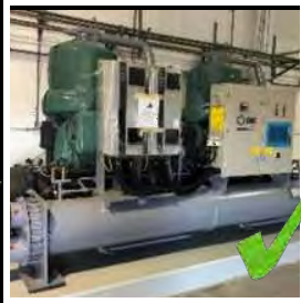
VAB ECS COMMISSIONING COMPLETE - READY FOR ML1 MEVV
