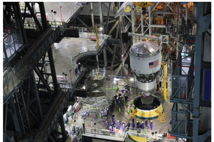
The interim cryogenic propulsion stage for the Artemis II SLS was added to the vehicle stack May 1.
