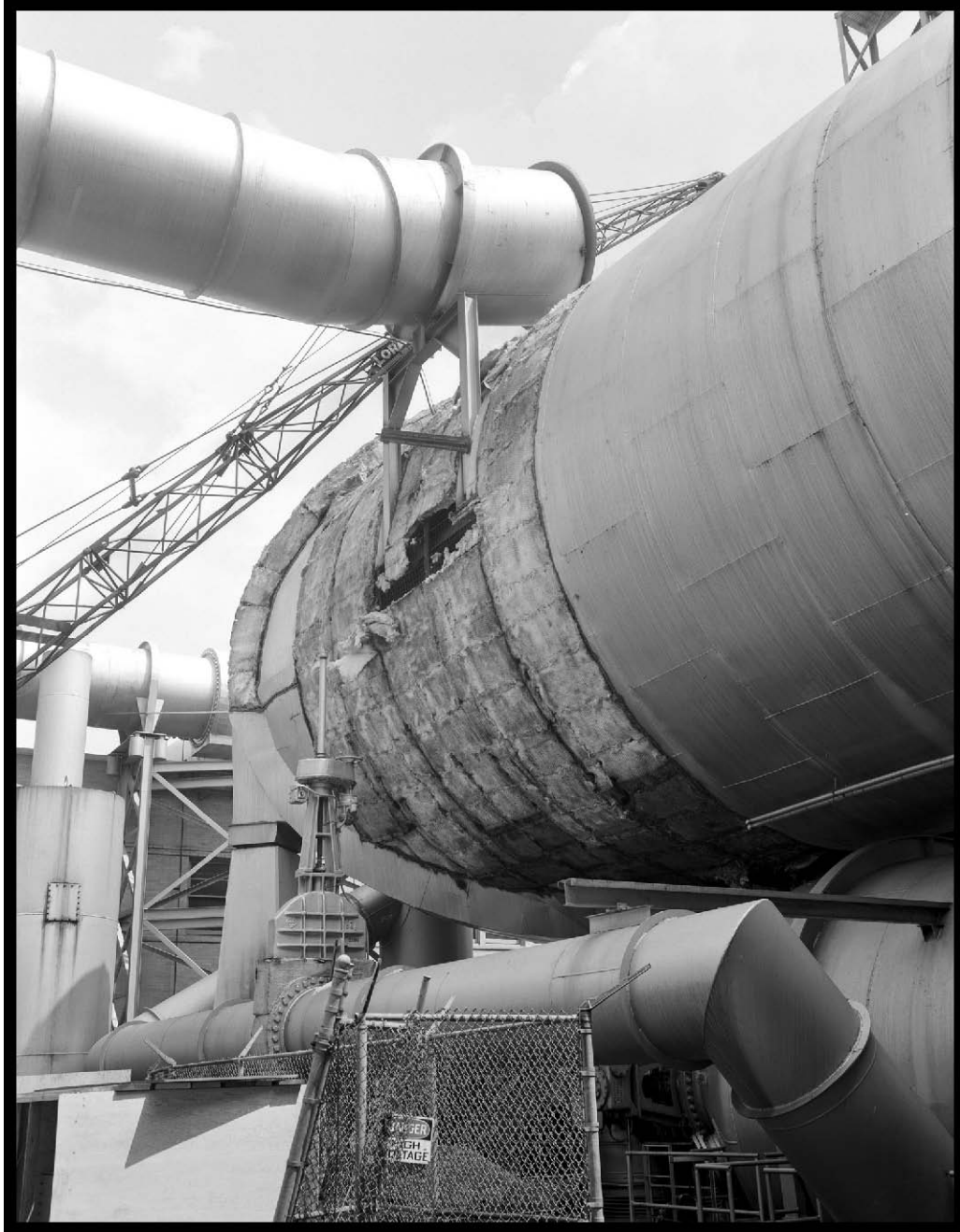
Figure 17.—Outer steel layer of the wind tunnel being removed so that the inner layer could be rewelded to create a higher vacuum seal, 1961 (OH_Cuyahoga_Space-Power-Chambers_017).
