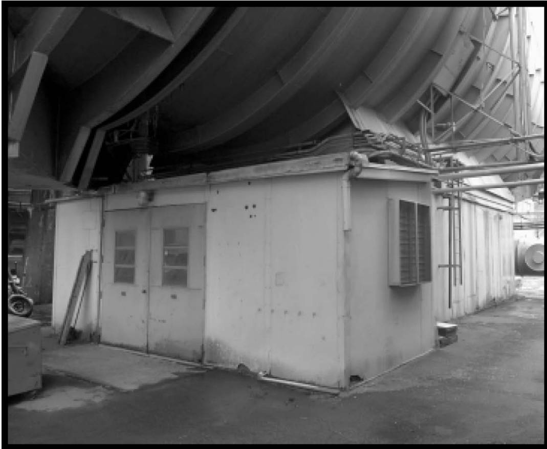
Figure 62.—Rear of Vacuum Pump House beneath SPC No. 1 (viewed from the southeast), 2007 (OH_Cuyahoga_Space-Power-Chambers_062).
