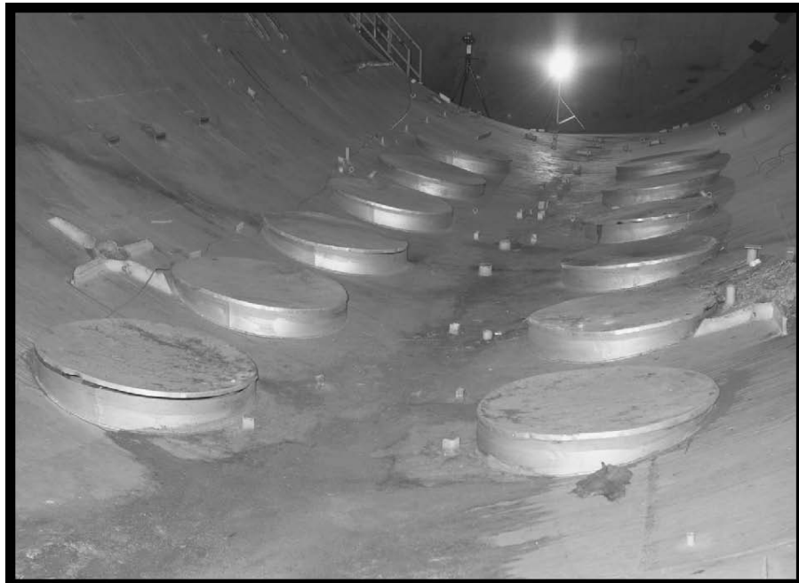
Figure 51.—SPC No. 1 floor showing water damage and numerous fittings from tests (viewed from the south), 2005 (OH_Cuyahoga_Space-Power-Chambers_051).
