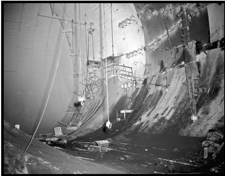
Figure 21.—Southwest corner of SPC No. 2 being renovated after the Project Mercury tests, 1961 (OH_Cuyahoga_Space-Power-Chambers_021).
