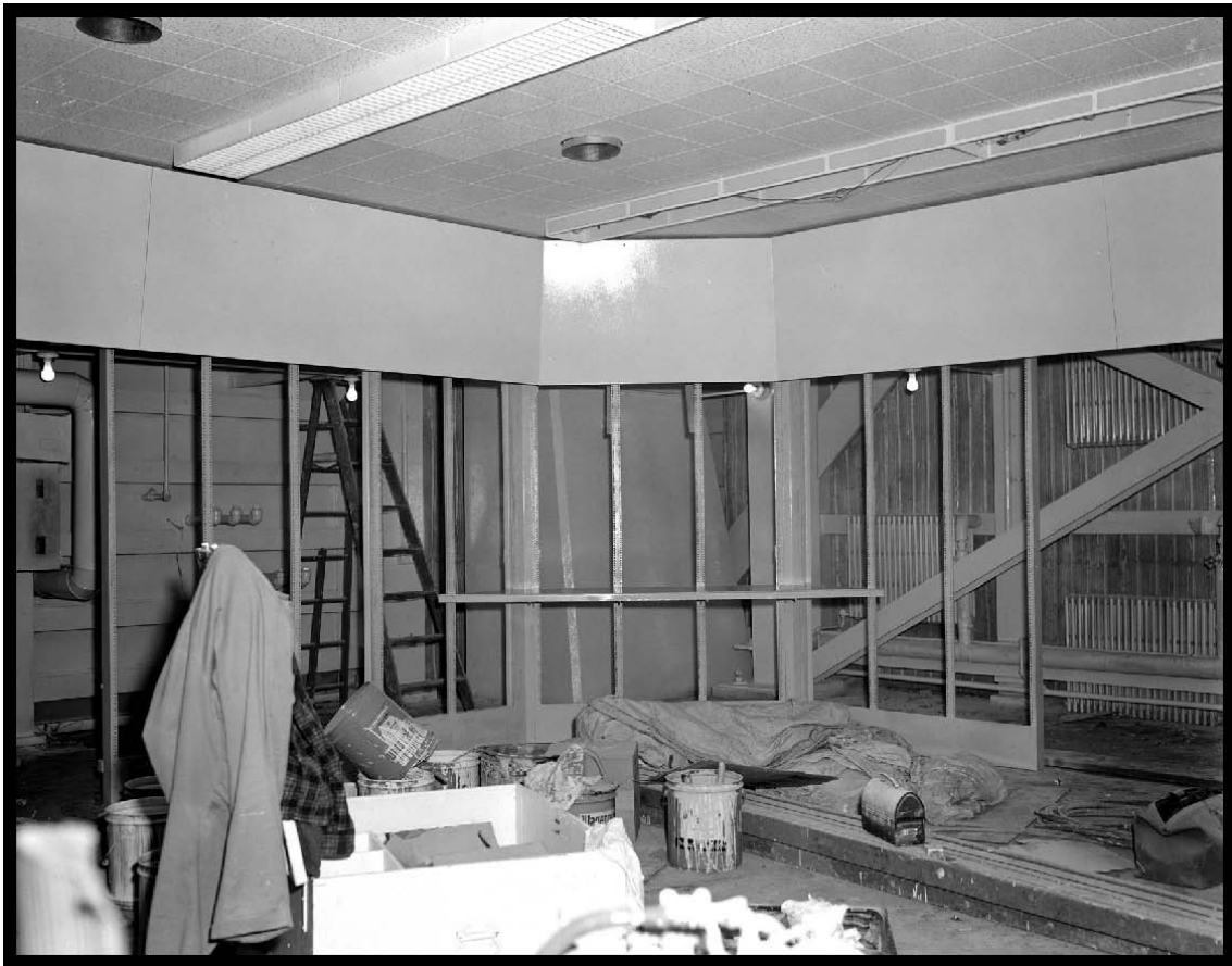
Figure 22.—Construction of the control room for the SPC underneath the former wind tunnel test section, 1961 (OH_Cuyahoga_Space-Power-Chambers_022).
