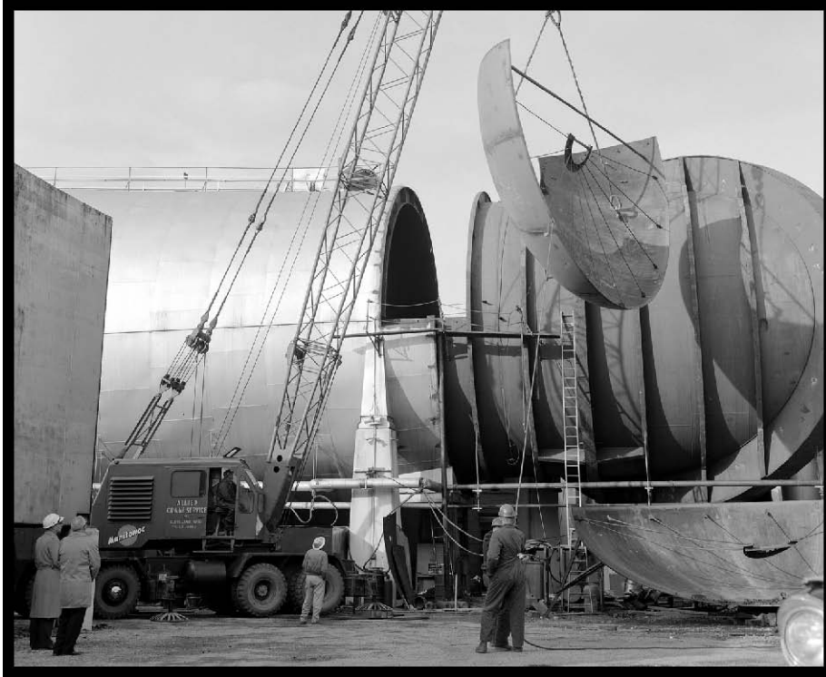
Figure 15.—Bulkhead section being lifted into the opening cut in the southeast corner of the tunnel, 1961 (OH_Cuyahoga_Space-Power-Chambers_015).
