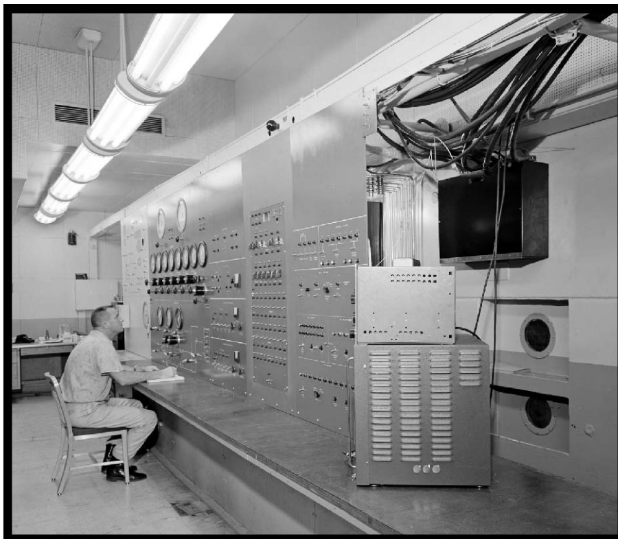
Figure 99.—SPC No. 2 control room (viewed from the west), 1963 (OH_Cuyahoga_Space-Power-Chambers_099).
