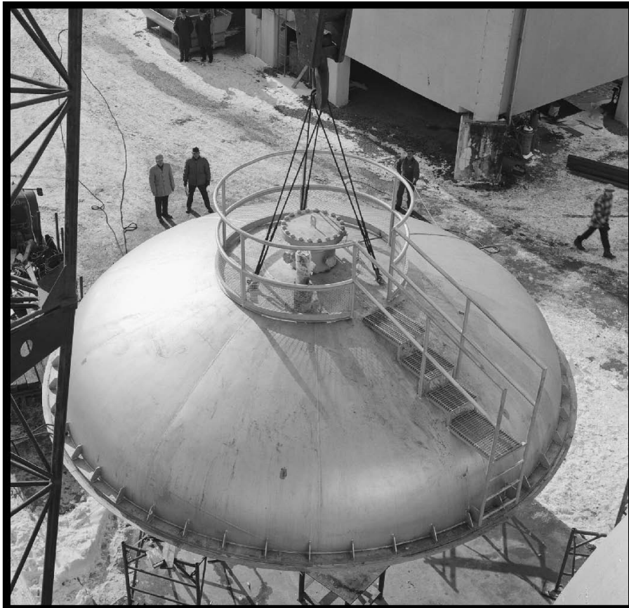
Figure 48.—SPC No. 1 lid being lowered to the ground by a crane, 1964 (OH_Cuyahoga_Space-Power-Chambers_048).
