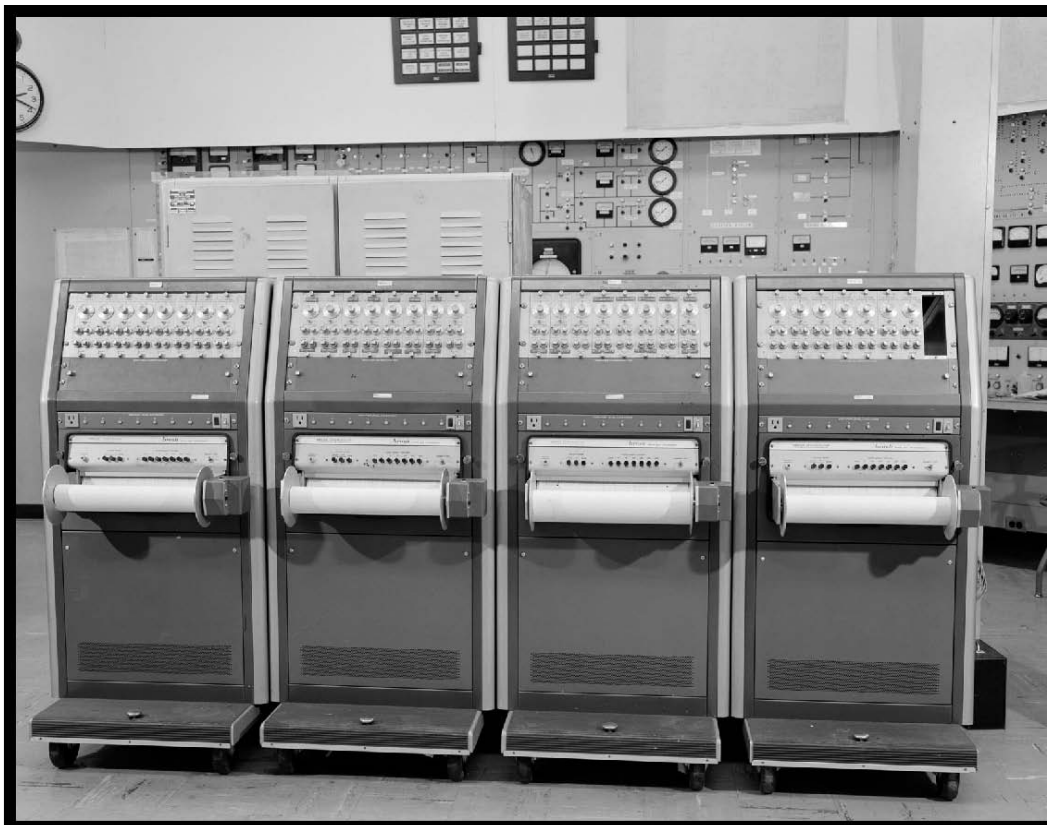
Figure 96.—Data recorders in the western rack in the center of the SPC No. 1 control room, 1967 (OH_Cuyahoga_Space-Power-Chambers_096).
