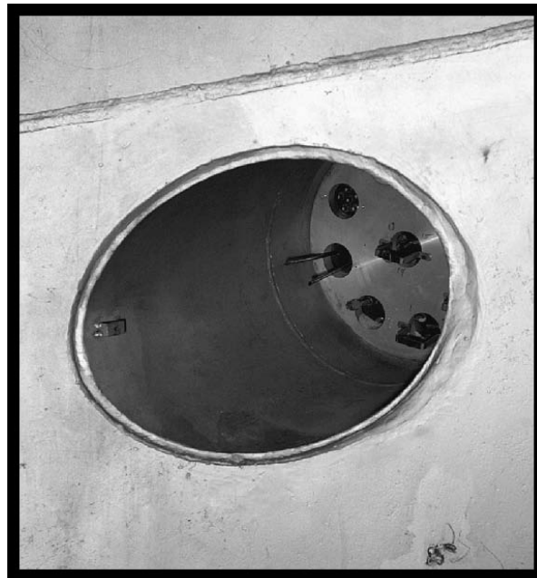
Figure 55.—Close-up of one of the instrumentation ports in the north SPC No. 1 bulkhead, 2005 (OH_Cuyahoga_Space-Power-Chambers_055).
