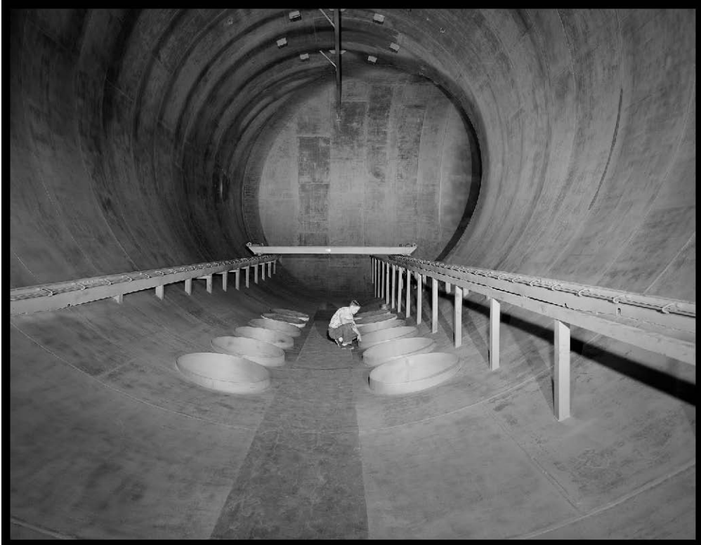
Figure 18.—Interior of SPC No. 1 prior to the addition of the dome, showing diffusion pump portals in the floor, 1962 (OH_Cuyahoga_Space-Power-Chambers_018).
