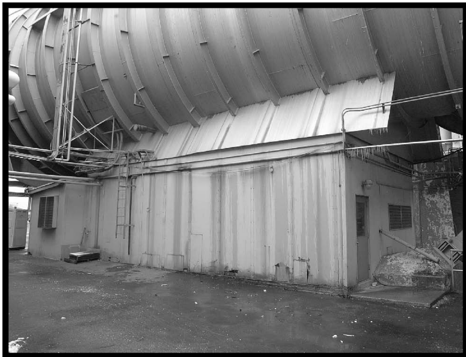
Figure 65.—Exterior of the Vacuum Pump House under SPC No. 1 (viewed from the northeast), 2007 (OH_Cuyahoga_Space-Power-Chambers_065).
