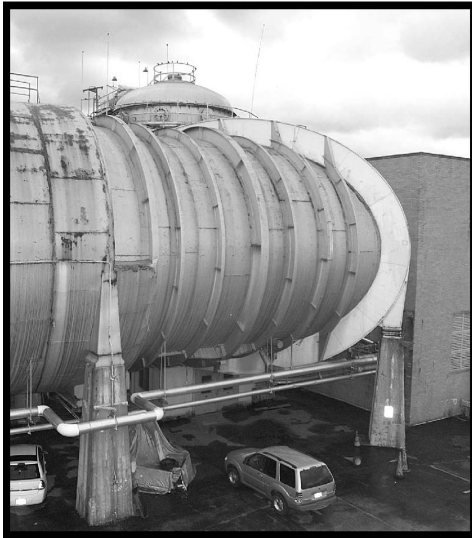
Figure 44.—SPC No. 1 shell to the right with the original tunnel outer shell to the left showing heavy rust damage, 2005 (OH_Cuyahoga_Space-Power-Chambers_044).
