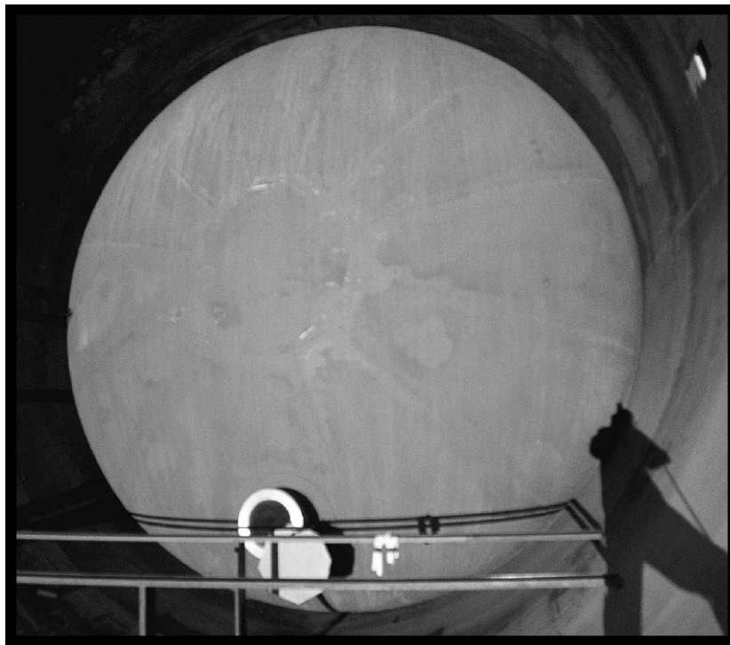
Figure 86.—31'-0"-diameter bulkhead near the southeast corner of SPC No. 2 (viewed from west of SPC No. 2), 2007 (OH_Cuyahoga_Space-Power-Chambers_086).
