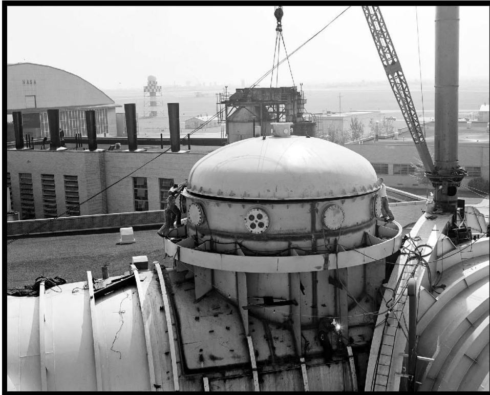
Figure 20.—Extension and dome created near the southeast corner of SPC No. 1 (viewed from the west), 1963 (OH_Cuyahoga_Space-Power-Chambers_020).
