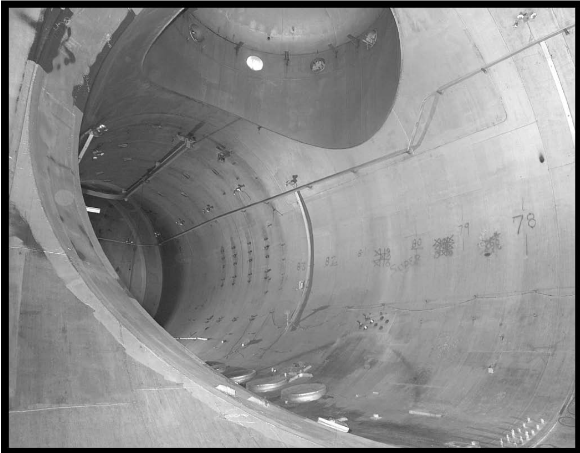
Figure 49.—SPC No. 1 interior with the extension and dome at the top and the cable tray along the wall (viewed from the north), 2005 (OH_Cuyahoga_Space-Power-Chambers_049).
