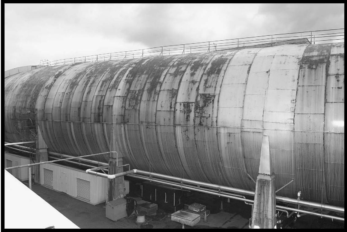
Figure 74.—South leg of SPC No. 2 with walkway on top (viewed from the south), 2005 (OH_Cuyahoga_Space-Power-Chambers_074).
