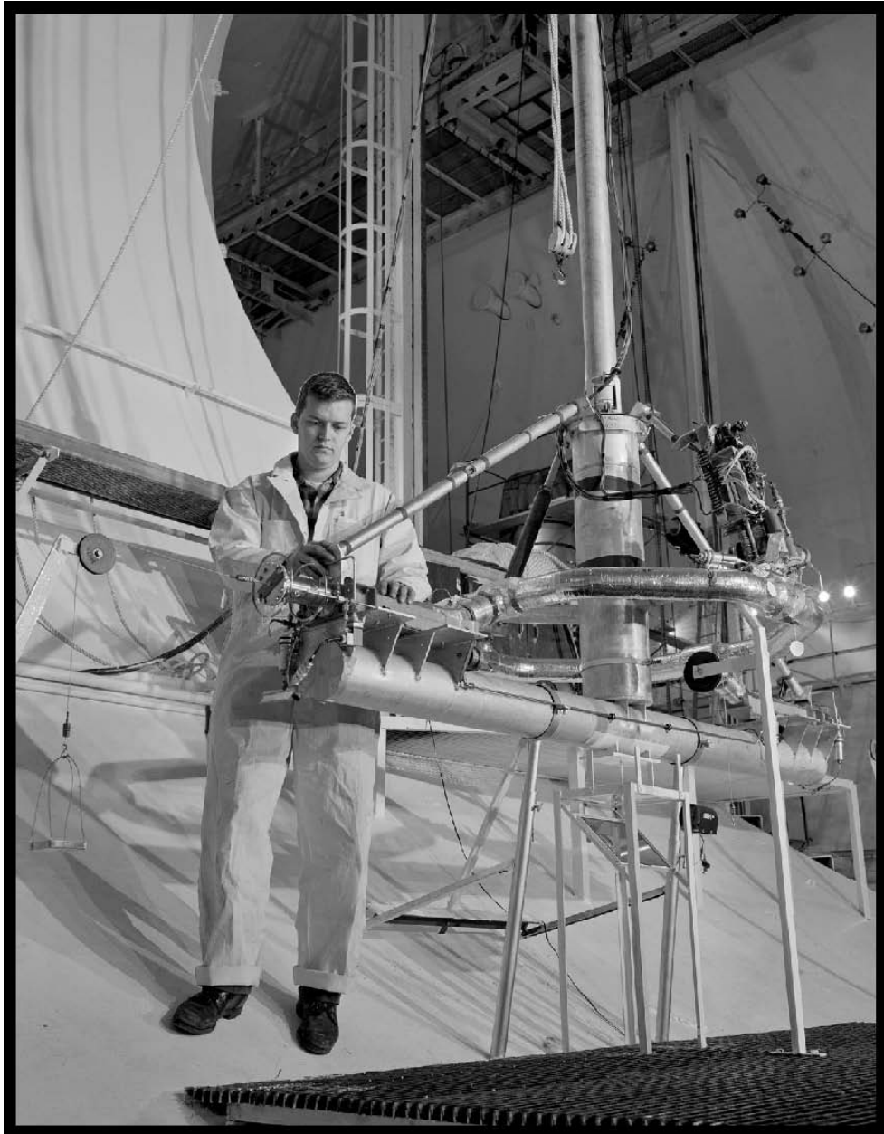
Figure 36.—Hydrogen vent rig installed in SPC No. 2 following the failure of the AC-4 flight because of sloshing, 1965 (OH_Cuyahoga_Space-Power-Chambers_036).
