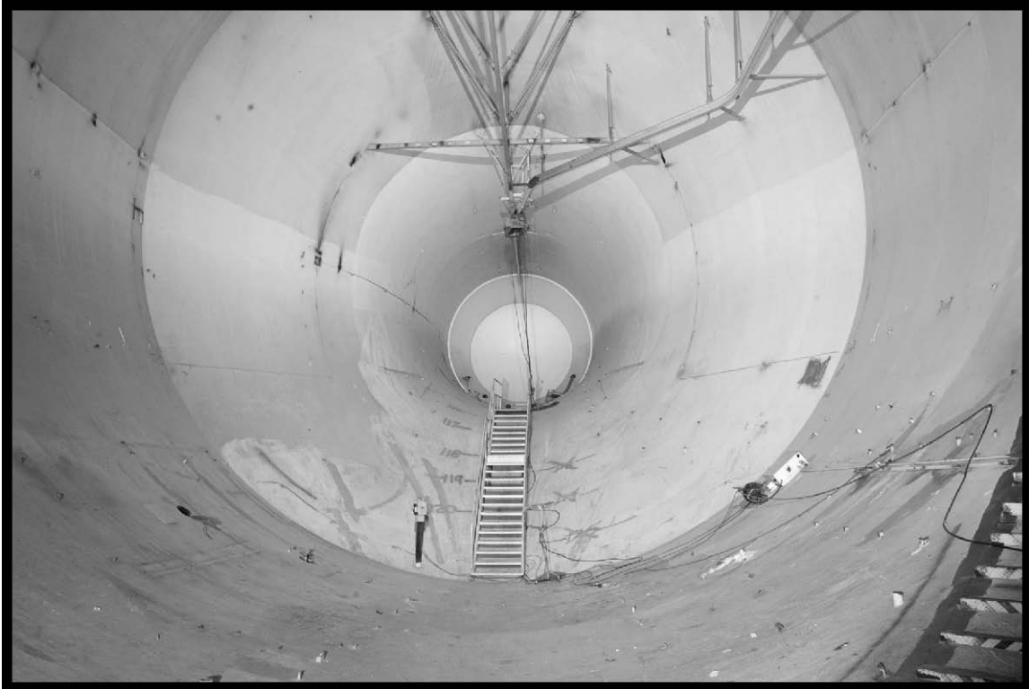
Figure 81.—Throat section of SPC No. 2 with the bulkhead at the far end (viewed from the west), 2007 (OH_Cuyahoga_Space-Power-Chambers_081).
