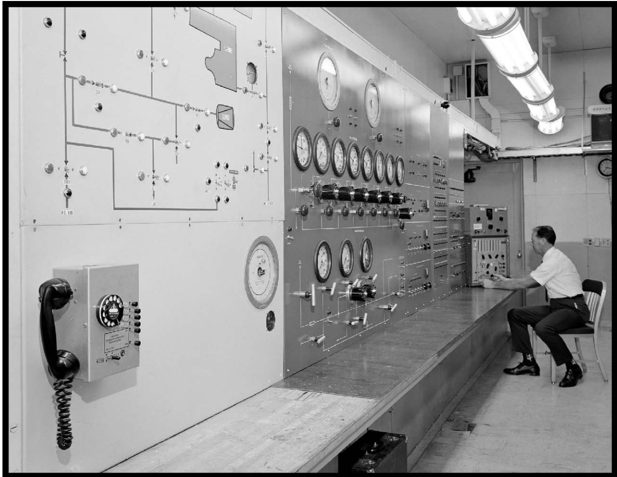
Figure 97.—SPC No. 2 control room with the airflow control panel in foreground (viewed from the east), 1963 (OH_Cuyahoga_Space-Power-Chambers_097).
