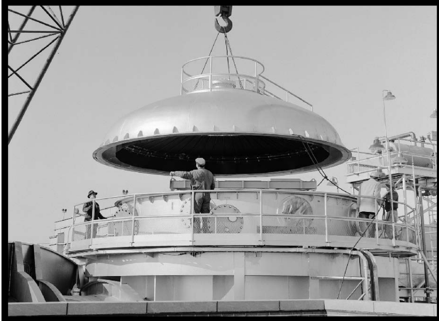
Figure 47.—Crane removing the lid from the SPC No. 1 dome (viewed from the east), 1964 (OH_Cuyahoga_Space-Power-Chambers_047).
