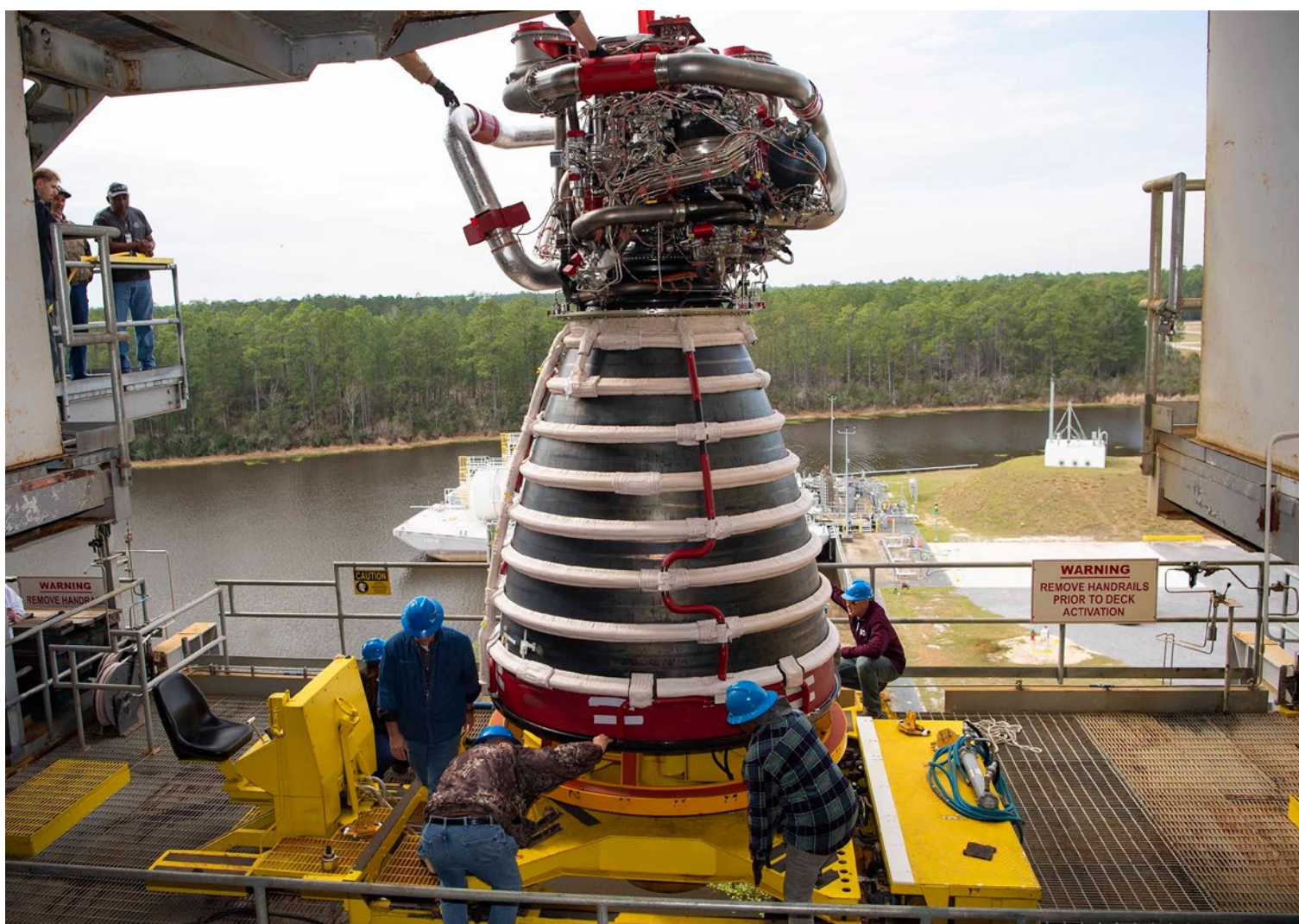
Teams at NASA's Stennis Space Center in Bay St. Louis, Mississippi, deliver, lift, and install the first new production RS-25 engine on the Fred Haise Test Stand on Feb. 18.
