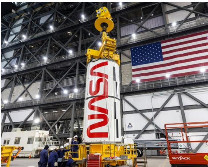
Engineers and technicians with NASA's Exploration Ground Systems Program prepare to lift the left center center booster segment shown with the iconic NASA "worm" insignia for the agency's SLS (Space Launch System) rocket in the Vehicle Assembly Building at NASA's Kennedy Space Center in Florida in January.
