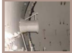
Make-Up Air Line
