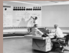
Central Control Room
