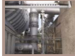
AWT Exhaust Pipe
