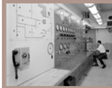
SPC No. 2 Controls
