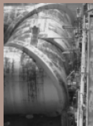
AWT Cooling Lines
