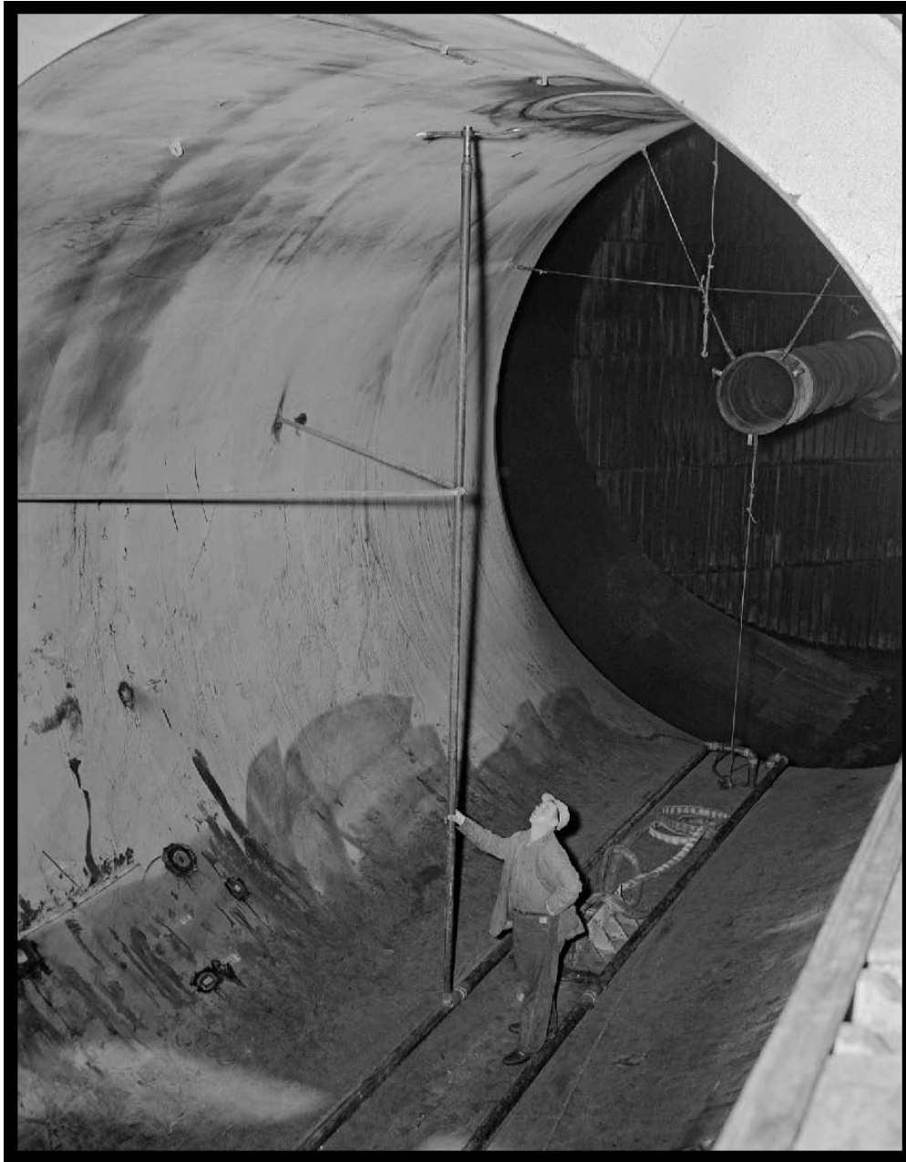
Figure 92.—Throat section and primary makeup air line of the AWT (viewed from the east), 1951 (OH_Cuyahoga_Altitude-Wind-Tunnel_093).
