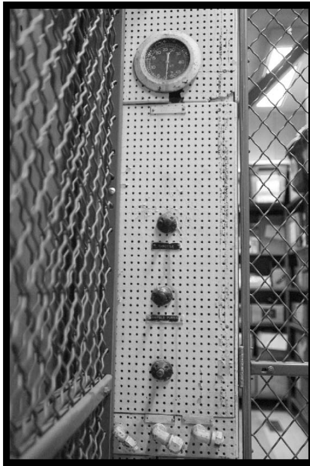
Figure 122.—Former AWT controls, 2007 (OH_Cuyahoga_Altitude-Wind-Tunnel_123).
