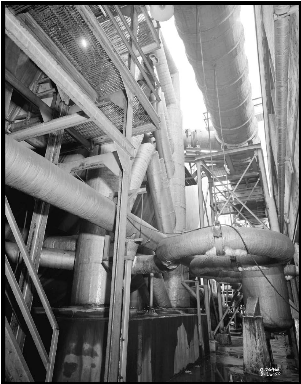
Figure 101.—Platform and cooling system pipes connecting the AWT (left) and the Refrigeration Building (right) (viewed from the north), 1950 (OH_Cuyahoga_Altitude-Wind-Tunnel_102).
