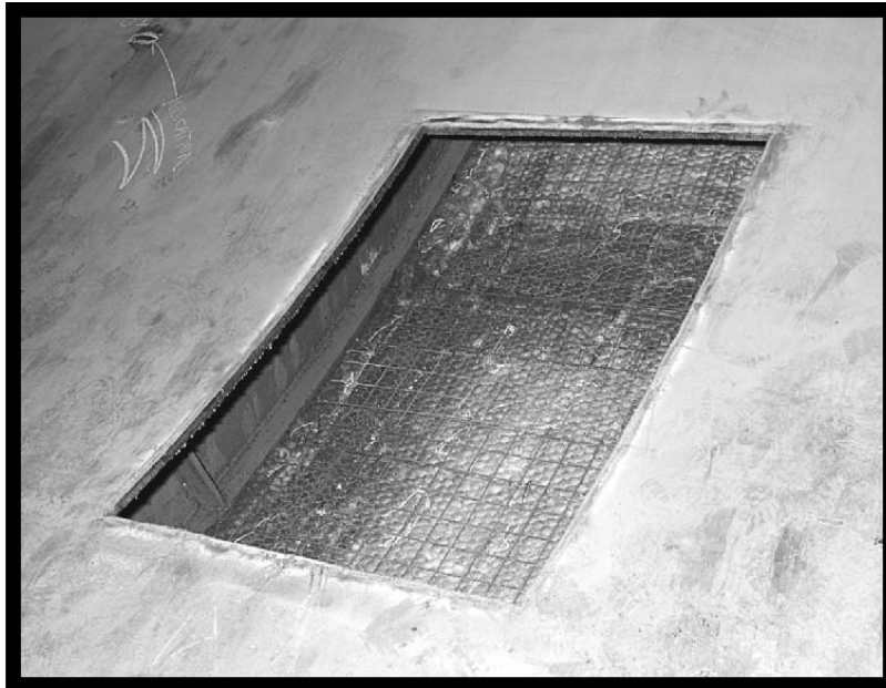
Figure 69.—One of a series of holes cut into the southern leg showing the tunnel's shells, mesh, and insulation, 2005 (OH_Cuyahoga_Altitude-Wind-Tunnel_070).
