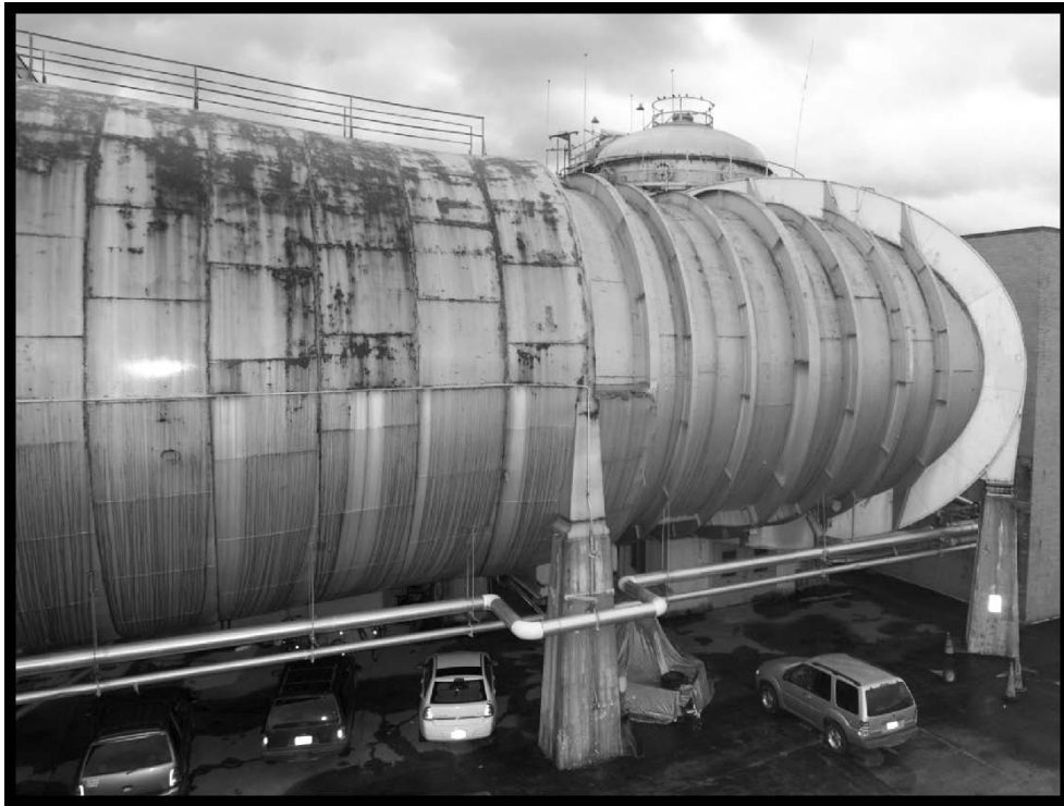
Figure 63.—Southeast corner of the AWT showing rust outlining the outer shell's square steel panels, 2005 (OH_Cuyahoga_Altitude-Wind-Tunnel_064).
