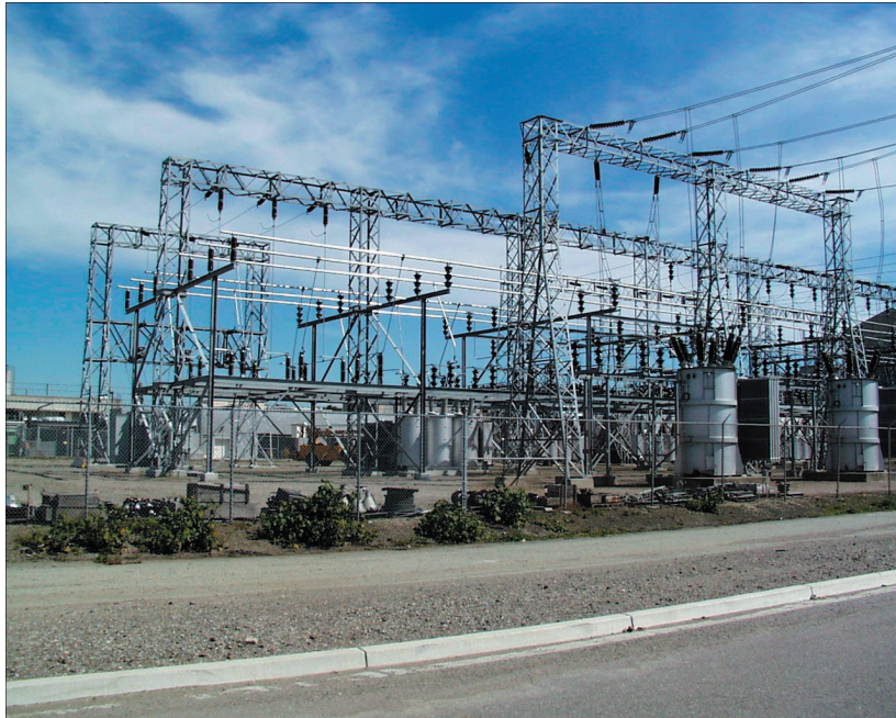
Ames Research Center Substation North
