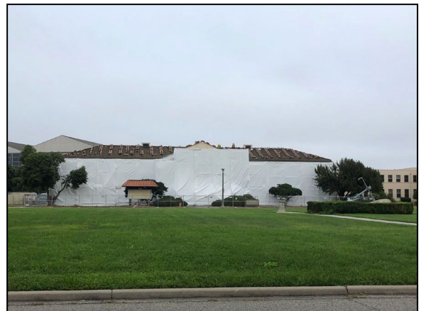
Figure 4-6. Exterior asbestos containment at Building 25.
