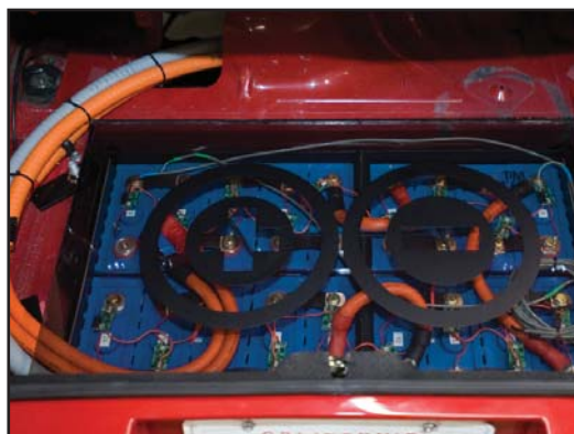
Rear battery pack in KleenSpeed Eiata trunk provides 10.5 kWh, with room for golf clubs or suitcase. KleenSpeed Eiata has two battery packs (one in front and rear) for balance, each comprised of 18 prismatic lithium ferrous phosphate cells.
