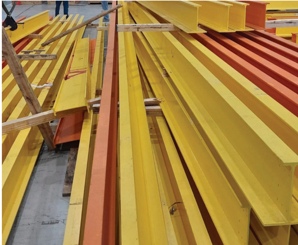
Figure 10: View of collapsed beams and broken dunnage.
