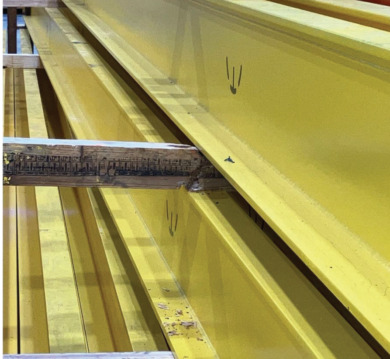
Figure 16: Fractured dunnage is re-mated to show position and fracture site.
