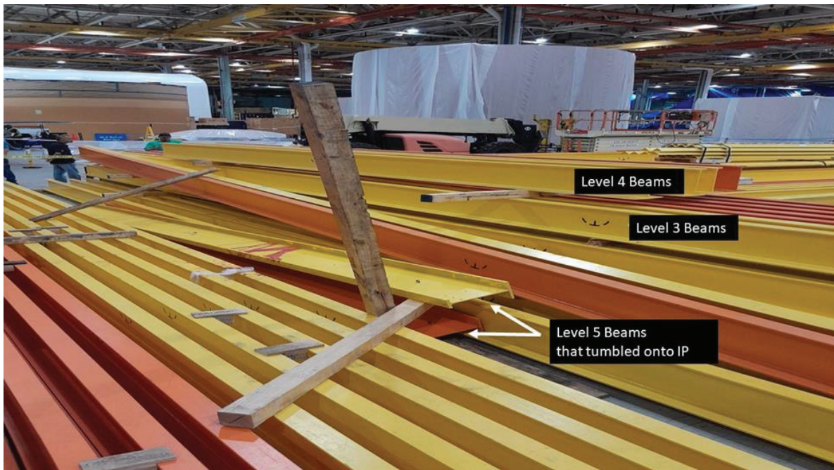
Figure 19: Beams from level 5 that tumbled onto IP, and beams that collapsed with breakage of dunnage.
