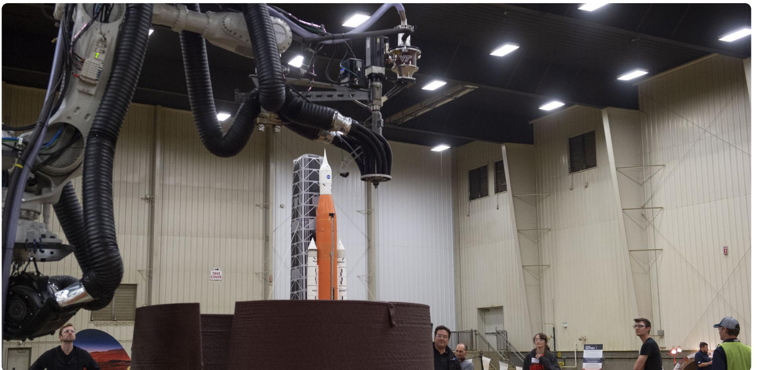
Team AI SpaceFactory's printer autonomously inserts a window into their 3D-printed subscale habitat structure at NASA's 3D-Printed Habitat Challenge, held at the Caterpillar Edwards Demonstration & Learning Center in Edwards, Illinois, May 1-4, 2019 Credits: NASA
