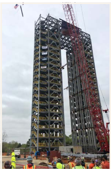
FIGURE 4. LH2 Tank Test Stand
