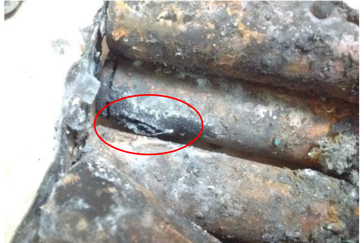
Not 100% reliable separation. Cells can vent outside of side casing
