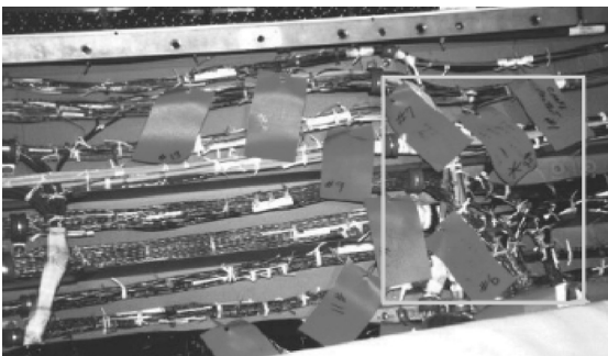
Figure 20 -- Close-up OV103 Mid-Body: Compromised Redundancies, Possible Chafing
