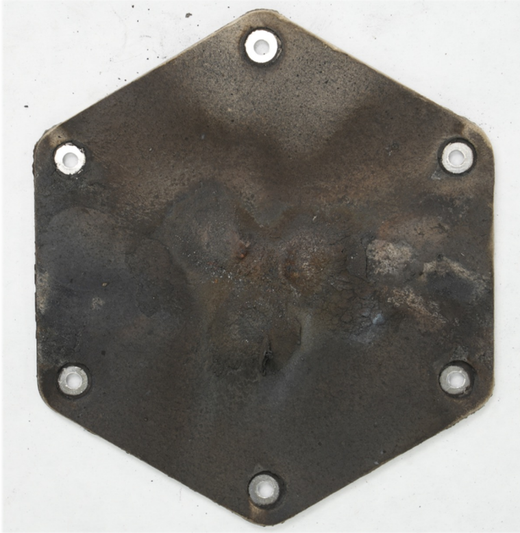
Figure: blast plate removed from positive end of battery – note buildup of cell ejecta aligned with trigger cells.
