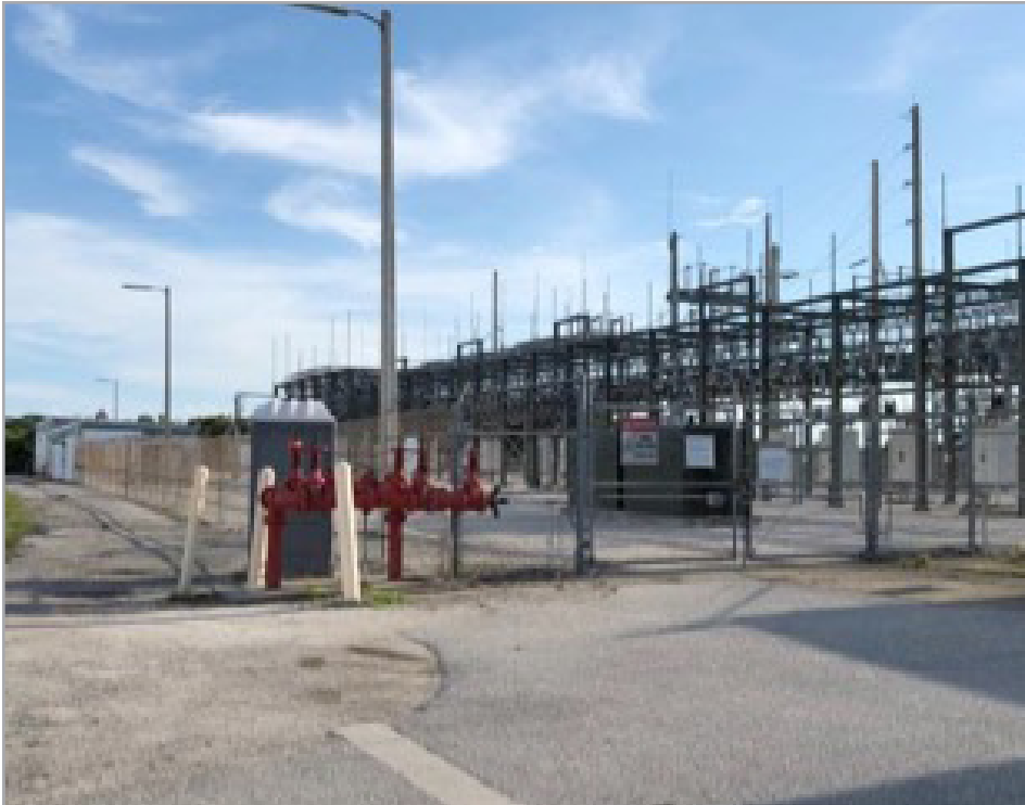
C5 Substation, Kennedy Space Center
