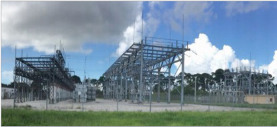
Orsino Substation, Kennedy Space Center
