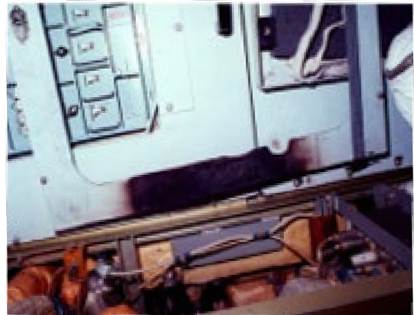
Damage after the Apollo 1 fire
