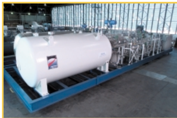
Propellant densification system at GRC.
