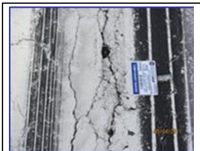
Section of Runway at Wallops Flight Facility Deteriorated Pavement in Centerline. This deteriorated pavement is typical of the condition at runways and taxiways throughout the airfield. NASA intends to correct the most severe pavement with an FY 15 Airfield Repair project. Additional work will be required in a second phase in the near future.
