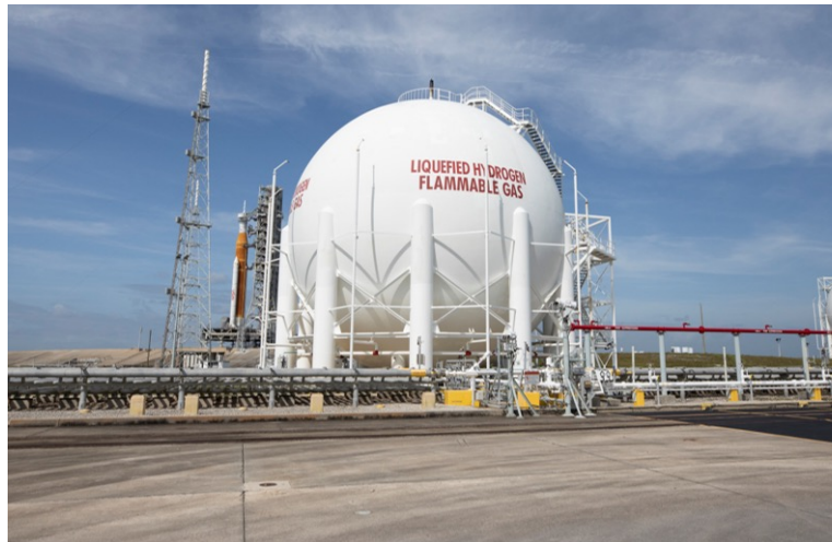
LH2 Tank at KSC
