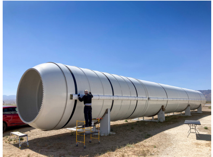
Installing SRB systems tunnels at the Mojave Air and Space Port where the motors are stored.
