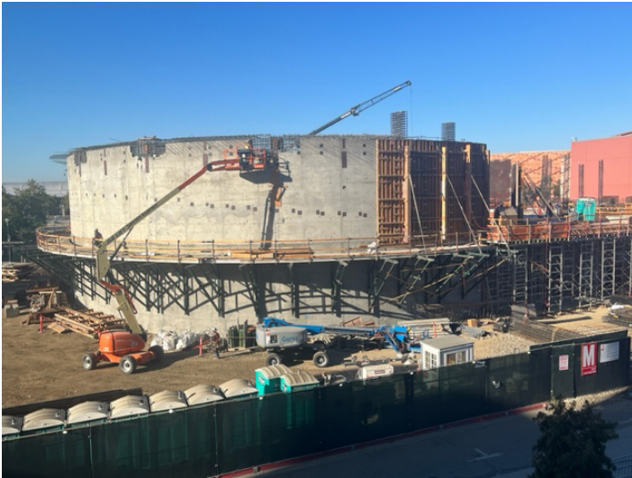
The Shuttle gallery as viewed from the north, showing the 42-foot-high concrete wall. There will be an additional 160 feet of structural steel placed above the wall to complete the Shuttle gallery.
