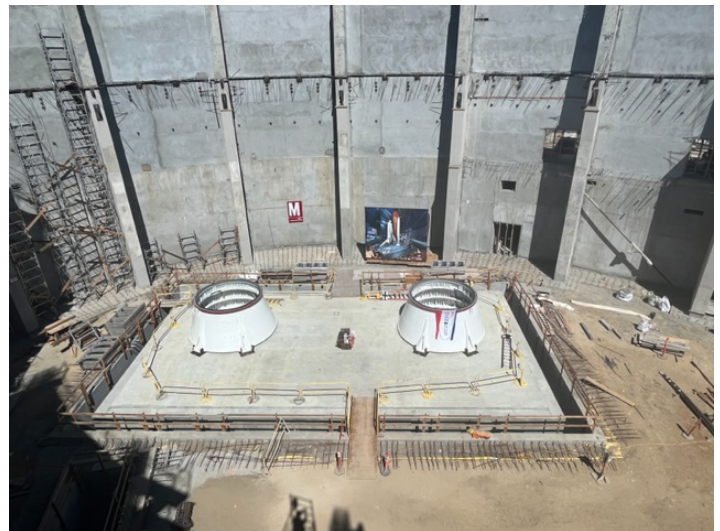
The aft skirts sitting on the isolation pad. Over the next couple of weeks, they will be extensively surveyed to make certain they are in the correct position and perfectly level. Then workers will install 9-foot-long inconel hold-down posts and torque them to 500,000 foot-pounds of torque (as a reference, the lug nuts on car wheels are typically about 110 foot-pounds).
