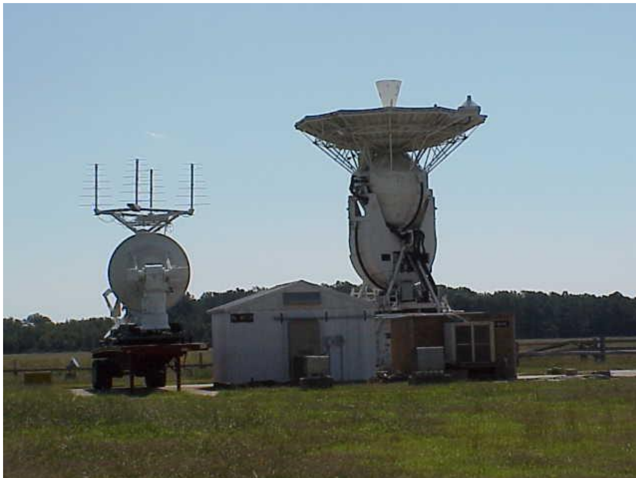
Figure 10.1.6-1: WFF Fixed Radar System
