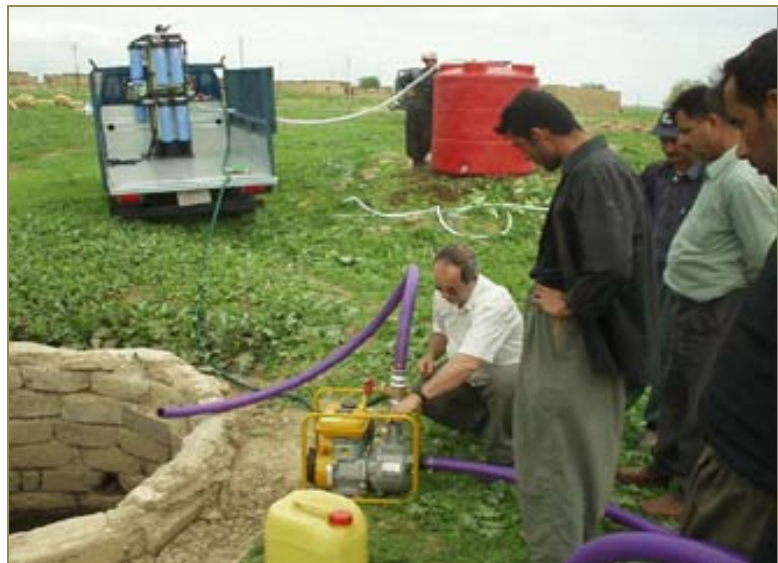
Volunteers help install and test a water purification system in Kendala, Iraq. (Image courtesy of Concern for Kids)
