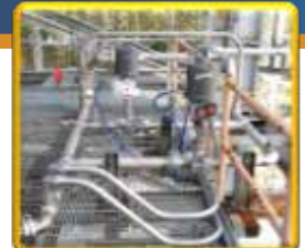
Cryogenic System Vent
