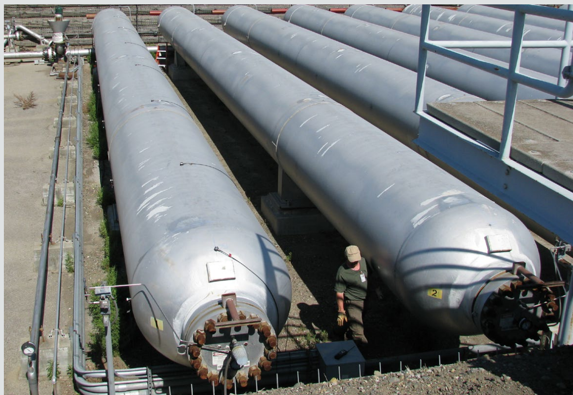
Typical large facility layered pressure vessels can be pressurized to 5,000 psi.
