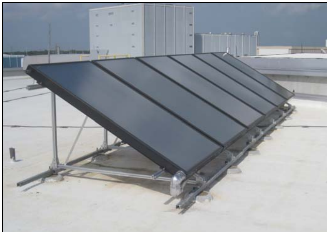
Figure 12 - Rooftop Solar Hot Water Heating System, Building 20, Johnson Space Center
