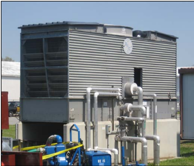
Figure 12 - Cooling Tower, Building 1238B, Langley Research Center
