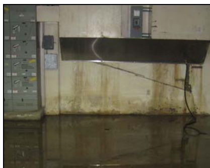
Figure 11 - Water Infiltration into Basement, Building 1298, Langley Research Center
