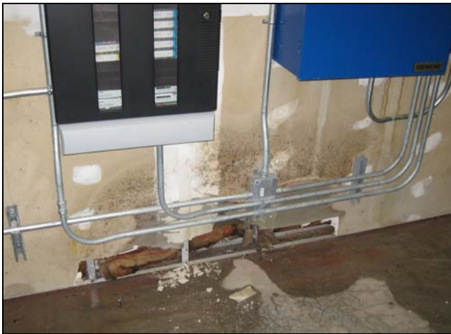
Figure 10 - Water Pipe Leak and Mold/Mildew Growth, Building 1210, Stennis Space Center
