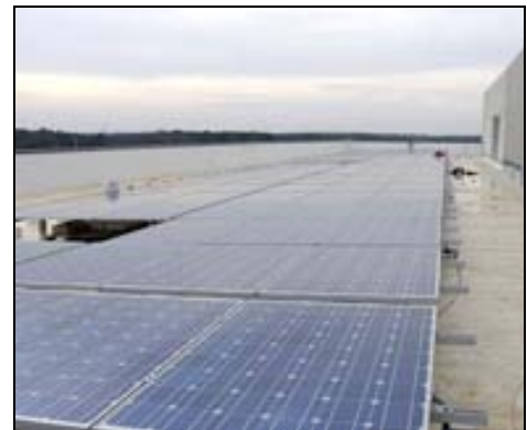
Figure 8 - Rooftop Solar Photovoltaic System, Marshall Space Flight Center
