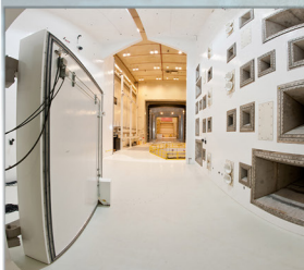
Reverberant Acoustic Test Facility
