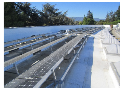
Figure 5 – Photovoltaic Panel Array
