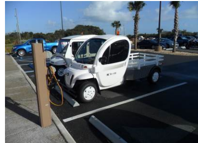
Figure 7 - Charging Station for Electric Vehicle
