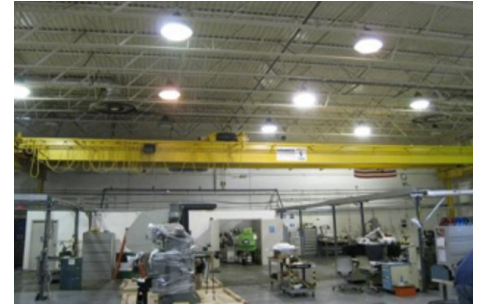
Affixed Overhead Crane
