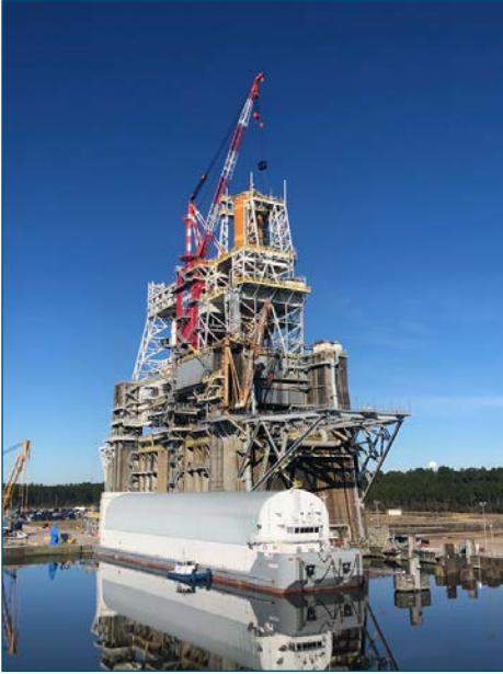
Pegasus moored at the Stennis Space Center B-2 Test Stand with the Core Stage installed in the test stand
