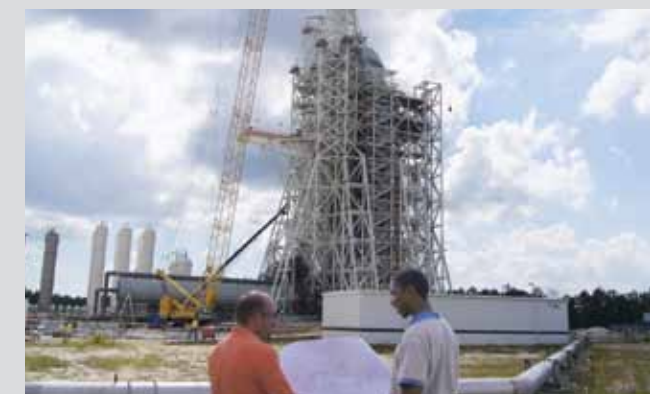
Jody Woods, A-3 Chief Engineer (left), and Dr. Howard Conyers, structural analyst, examine plans for the signal conditioning building, shown in the foreground of the A-3 test stand.
