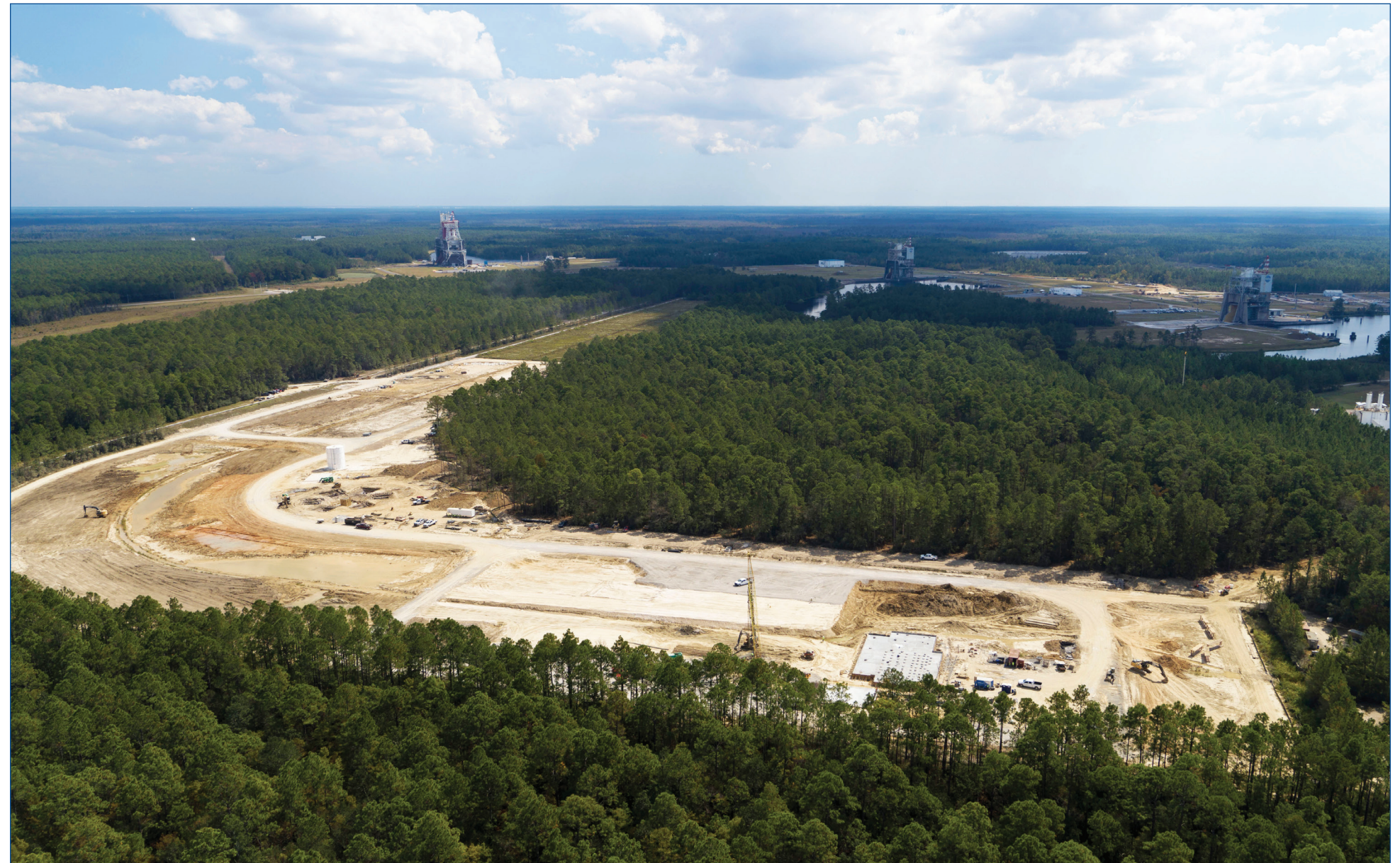
An aerial image shows a cleared area at NASA's Stennis Space Center where Relativity Space plans to build several new test-related facilities. The aerospace company is substantially expanding its presence at Stennis
