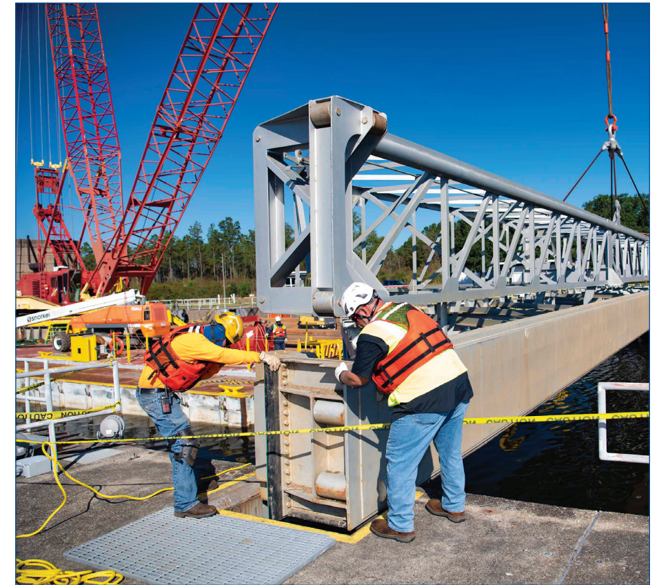
Crews position stop logs to ensure the canal system that connects NASA's Stennis Space Center to the Pearl River will maintain the proper water level as gates to the navigation lock system undergo upgrades.
