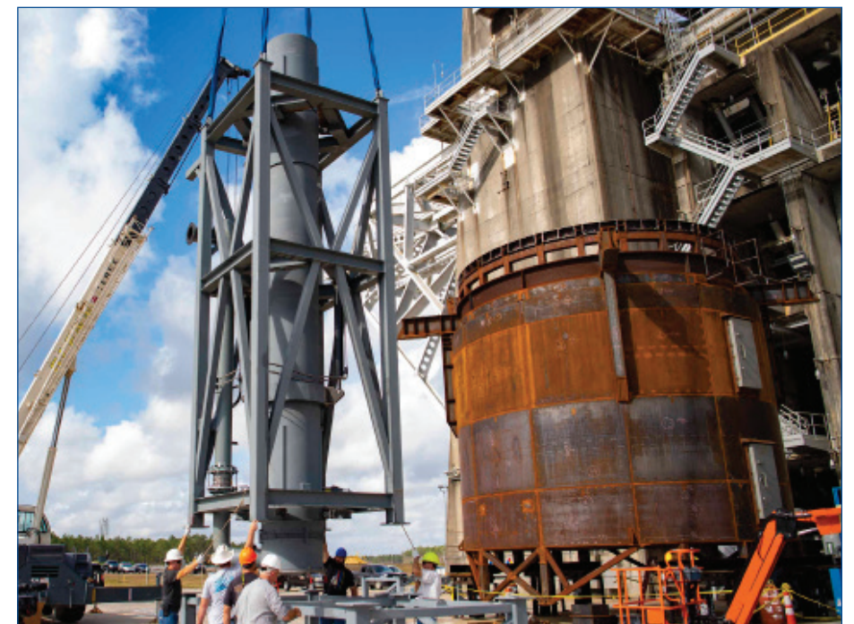
NASA Stennis crews adjust a diffuser module at the B-2 Test Stand following the arrival of the modules on Dec. 6, 2022. Modifications at the B-2 Test Stand will continue in 2023 for future Green Run testing of the Exploration Upper Stage.
