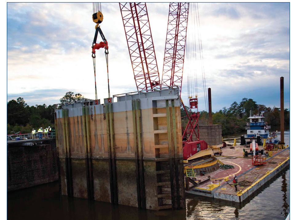
Crews use a crane on a floating barge to lift the lower south gate of the navigation lock system at NASA's Stennis Space Center on Nov. 21. The four gates, each weighing 270,000 pounds, were taken off site to undergo full inspection and refurbishment.
