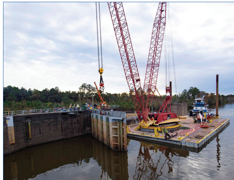
Crews remove the lower south gate to the navigation lock system at NASA's Stennis Space Center using a crane on a floating barge on Nov. 21. A months-long project is underway to ensure essential lock access continues as the site supports NASA's mission to explore the secrets of the universe for the benefit of all.
