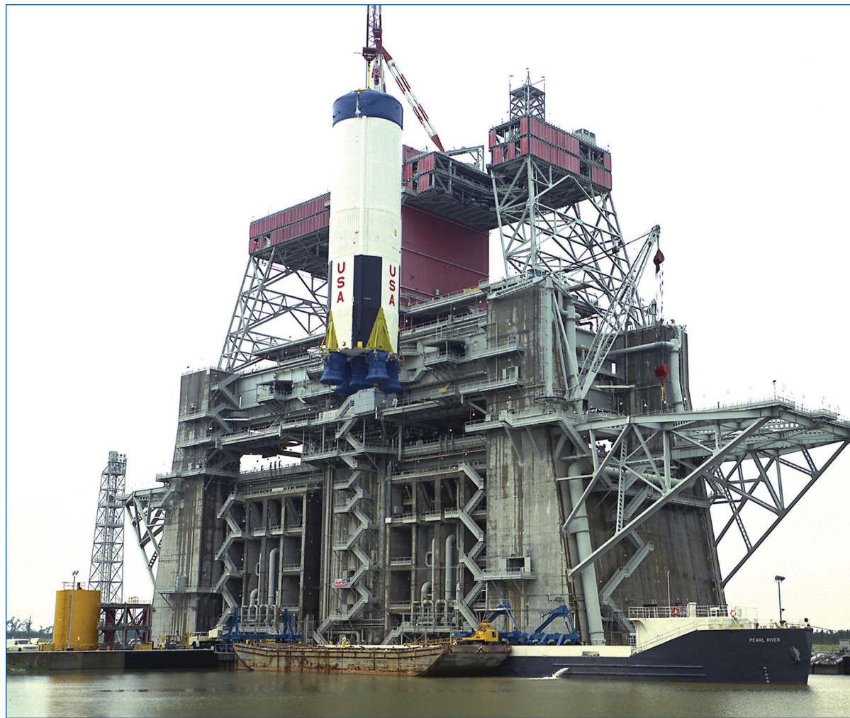
A derrick crane lifts the Saturn V S-IC-12 onto the B-2 Test Stand at NASA's Stennis Space Center on July 18, 1969, in preparation for hot fire testing and use on the final Apollo 17 mission to the Moon.
