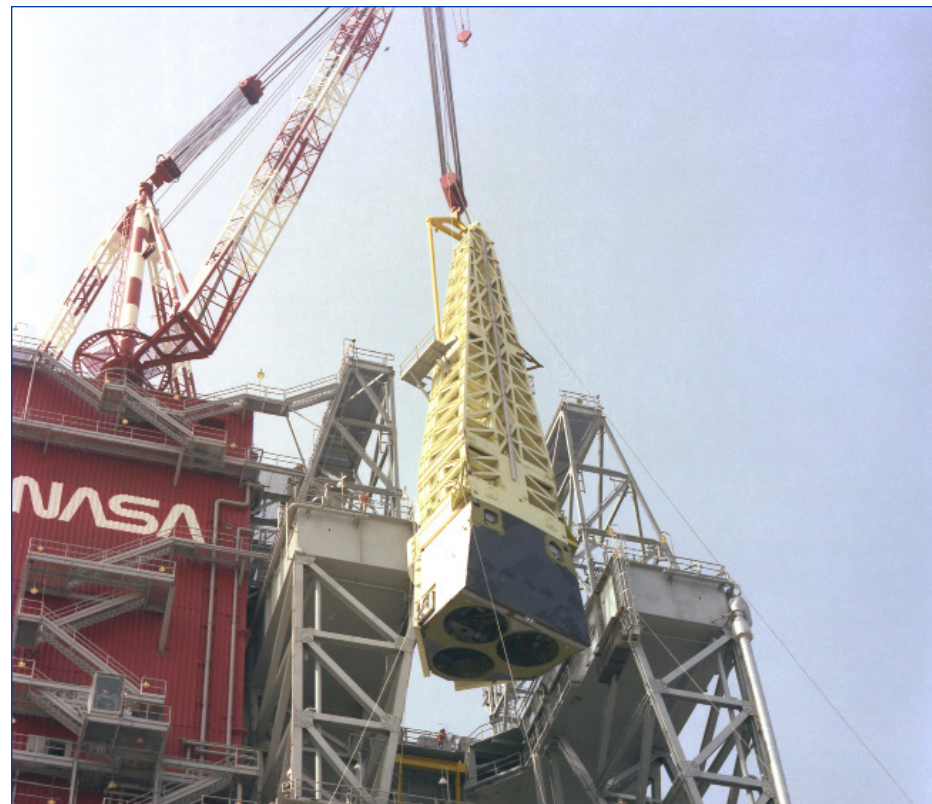
A space shuttle main propulsion test article (MPTA) component is lifted onto the B-2 Test Stand at NASA's Stennis Space Center, then known as National Space Technology Laboratories, in this 1977 photo. MPTA testing involved installing a shuttle fuel tank, a mockup of the shuttle orbiter, and the vehicle's three-engine configuration on the stand, then firing all three engines simultaneously, as would be done during an actual launch.
