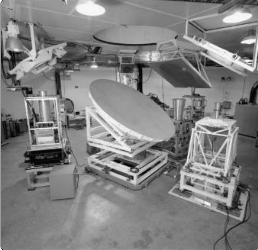
Figure 7-6. Stationary equipment room below the BWG antenna.
