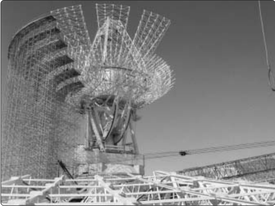
Figure 4-16. Work in progress on the 60-m-to-70-m antenna extension at DSS 14, Goldstone, December 1987.
