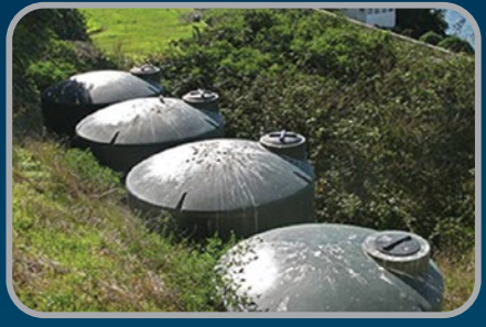
Parks use low-flow faucets and dual-flush toilets to conserve water. Parks use catchment tanks, like those pictured here, to collect and reuse rainwater. What can you do to help protect this precious resource?
