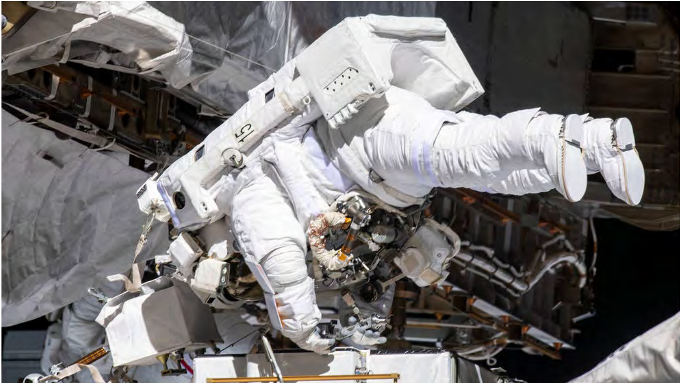
Astronaut Christina Loch works in the vacuum of space while tethered near the Port 6 truss segment of the International Space Station to replace older hydrogen-nickel batteries with newer, more powerful lithium-ion batteries, during the October 11, 2019, spacewalk. Fellow NASA astronaut Andrew Morgan (out of frame) assisted Koch during the six-hour and 45-minute spacewalk. Photo Credit: NASA
