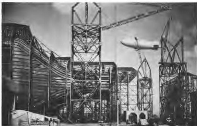
Above: June 24, 1943, 40- by 80-foot tunnel under construction, Navy Patrol blimp in background. Below: 40- by 80-foot tunnel completed, technical service building, utilities building, and 16-foot tunnel adjacent.
