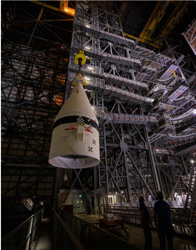
▲ In the transfer aisle of the Vehicle Assembly Building at NASA's Kennedy Space Center in Florida, workers use a crane to lift up the left-hand booster forward assembly for the agency's Space Launch System for transfer into High Bay 3 on March 1, 2021.
