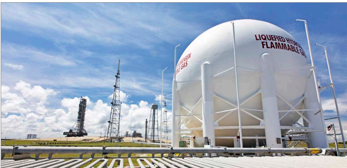
At Launch Pad 39B at NASA's Kennedy Space Center, liquid hydrogen tanks that supported Space Shuttle launches for 30 years have been sandblasted, repaired, and repainted. Along with the liquid oxygen storage vessel, the two tanks are designed to store super-cold propellants. They were refurbished to support NASA's Space Launch System rocket and other launch vehicles. (Photo credit: NASA)
