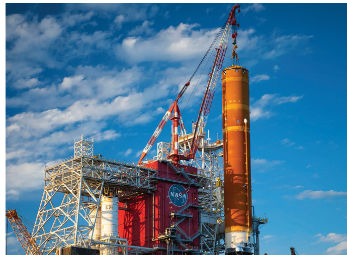
Artemis I core stage removal from B-2 test stand at NASA's Stennis Space Center following successful green run test.
