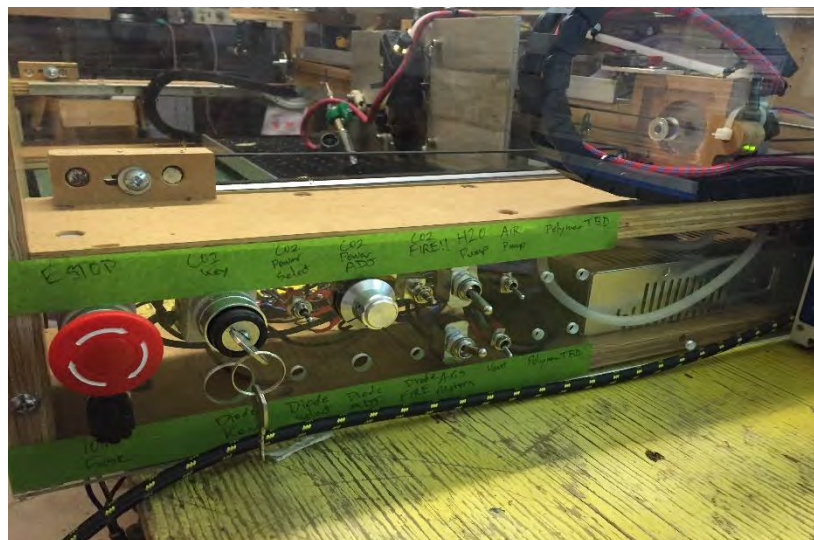
Figure: The control panel is shown above.
