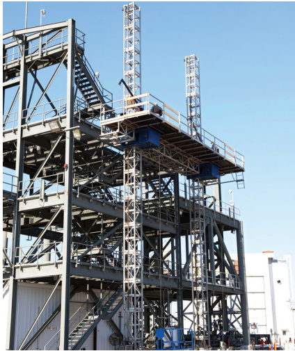
Workers receive training atop a mast climber that is attached to launch simulation towers outside the Launch Equipment Test Facility in February 2011. The training includes attaching carrier plates, water and air systems, and electricity to the climber to simulate working in Kennedy's Vehicle Assembly Building.
