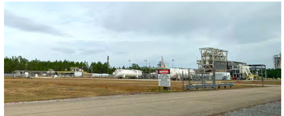
Supporting Infrastructure in the Test Complex Area
